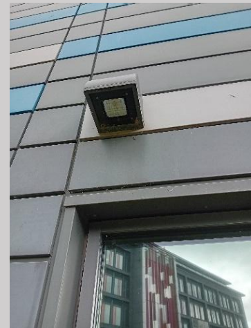
Photograph 16: Lighting block A.
