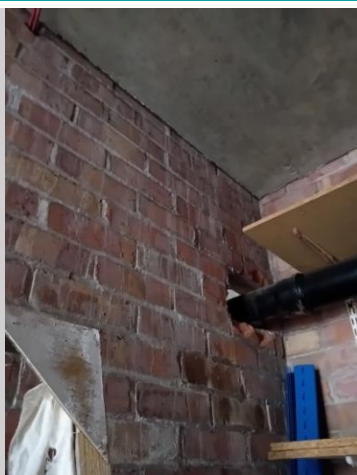
Photograph 25: Gaps were present in the internal walls between the garages.
