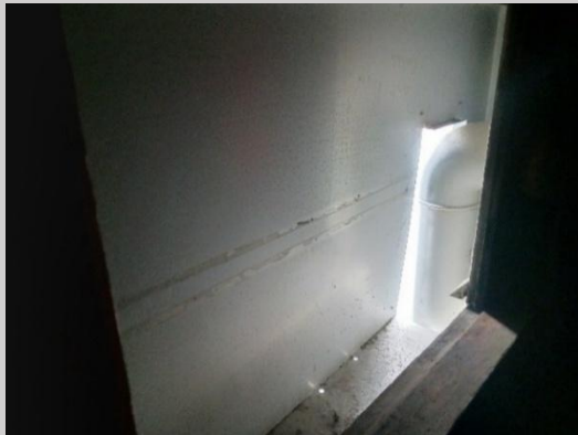
Photograph 21: Water tank room, block B. Potential access for bats.
