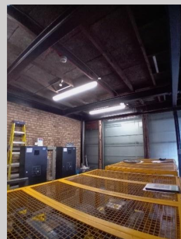
Photograph 18 Wiring room, block B.
