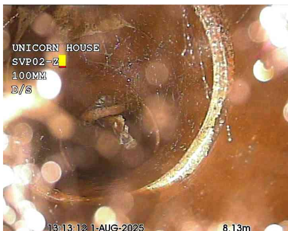
SVP02_3c0ea611-f695-43ce-85b2-98727351eb38_20250807_121906_317.jpg, 00:01:10, 8.13 m Hole in drain or sewer from 10 o'clock to 12 o'clock
