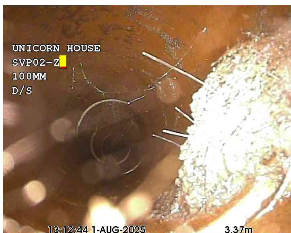
SVP02_79927a30-6b8b-4714-80bc-3506aa2776d1_20250807_121527_902.jpg, 00:00:42, 3.37 m Roots, mass at joint, 10% cross-sectional area loss
