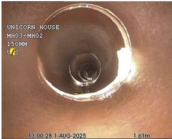
MH02_be9043b9-fd8c-464c-96f4-ea3db8010cdd_20250807_1 13543_314.jpg, 00:00:17, 1.61 m Joint displaced, medium
