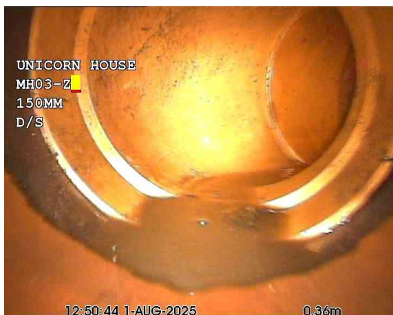
MH03_f2a53a16-d307-4303-af9e-4bc18c37c83c_20250807_11851_115.jpg, 00:00:05, 0.36 m Open joint, large
