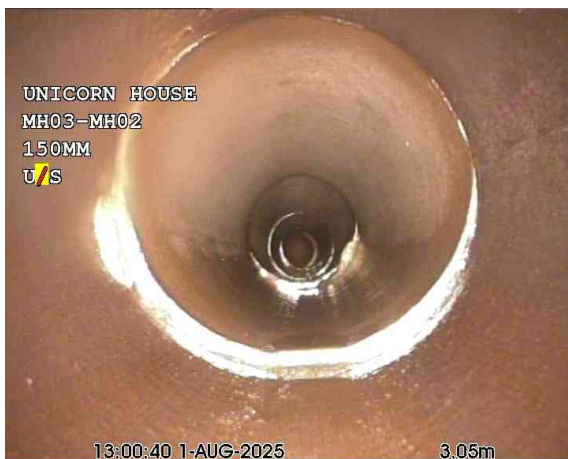
MH02_37f21446-291f-4885-ae03-5c3d8d025695_20250807_ 114105_401.jpg, 00:00:29, 3.05 m Joint displaced, medium
