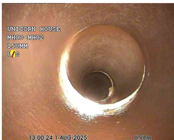
MH02_21c46e36-d9c8-4333-9de4-e9820aa89ad9_20250807_ 113448_887.jpg, 00:00:13, 0.98 m Joint displaced, large
