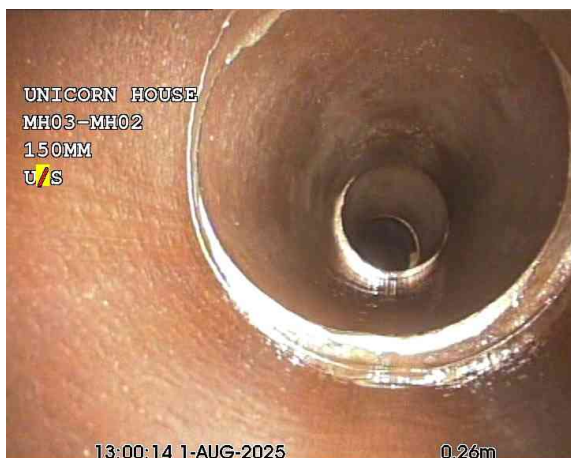
MH02_32e4e53f-4387-4807-a5fe-92f3601dc9b6_20250807_1 13249_977.jpg, 00:00:03, 0.26 m Crack, circumferential at joint from 7 o'clock to 12 o'clock
