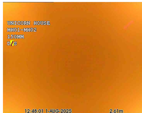
MH01_6af5c905-e9c1-43e6-b2c2-9376616de83b_20250807_ 111022_100.jpg, 00:00:26, 2.61 m Loss of vision, camera under water
