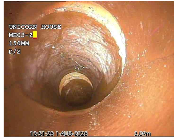
MH03_447b729e-dae9-42d3-9fbc-0116e534251f_20250807_112507_772.jpg, 00:00:53, 3.81 m Joint displaced, large
