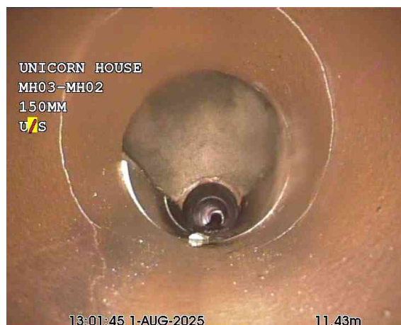
MH02_d530ed01-3a16-47c3-bc8c-5994f64a15b9_20250807_114925_957.jpg, 00:01:33, 11.43 m Crack, circumferential from 12 o'clock to 12 o'clock
