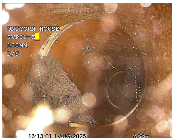
SVP02_5923512c-d3be-4a7d-b6e2-49a29d370f2b_20250807_121634_694.jpg, 00:00:59, 6.29 m Roots, mass at joint, 30% cross-sectional area loss
