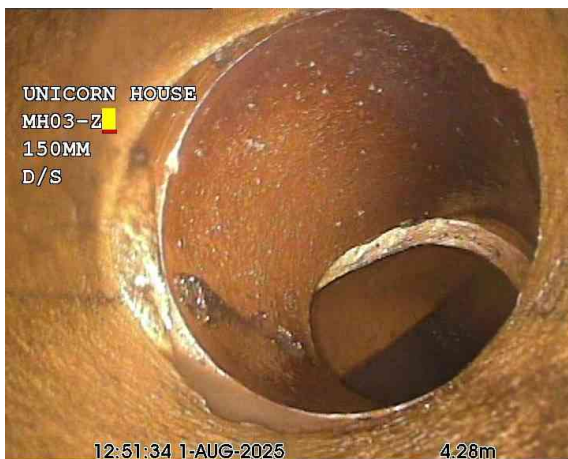
MH03_9013f87e-202b-407b-af11-55057019b937_20250807_112601_879.jpg, 00:00:55, 4.28 m Joint displaced, large
