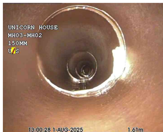
MH02_e4946c1f-7ccc-4114-b3ae-aeb7eb081feb_20250807_1 13520_417.jpg, 00:00:17, 1.61 m Crack, circumferential at joint from 12 o'clock to 12 o'clock
