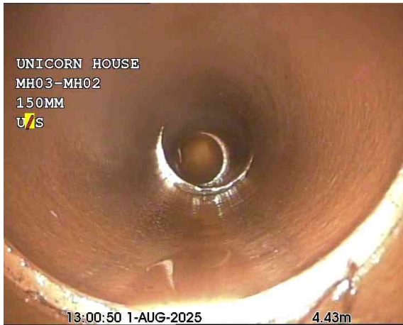
MH02_39153886-8e83-4fbf-90d9-0be98e1cdabc_20250807_114237_158.jpg, 00:00:39, 4.43 m Joint displaced, medium
