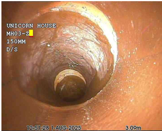
MH03_99c7ba3a-1cde-4992-a401-345e34a2d39e_20250807_112431_008.jpg, 00:00:49, 3.09 m Joint displaced, large
