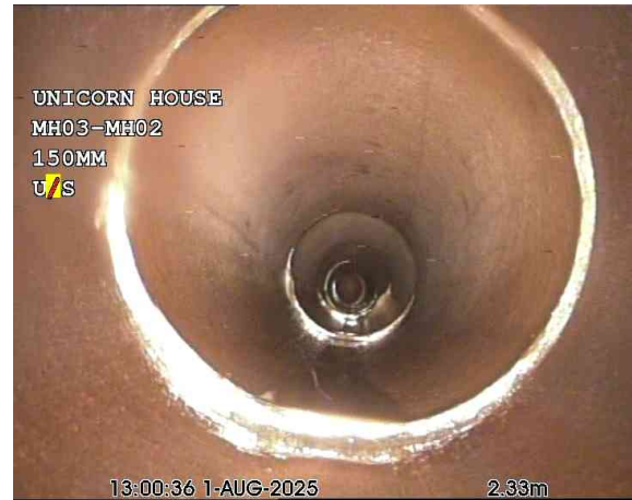
MH02_3dffb7e-d021-4f27-a150-a183a49be435_20250807_1 13609_855.jpg, 00:00:25, 2.33 m Joint displaced, medium
