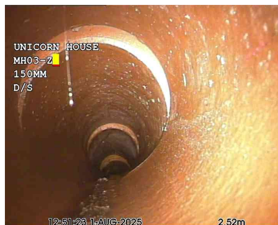
MH03_061212bb-9fde-4c68-a538-d0ce1ad9c9d0_20250807_112406_584.jpg, 00:00:44, 2.52 m Joint displaced, large
