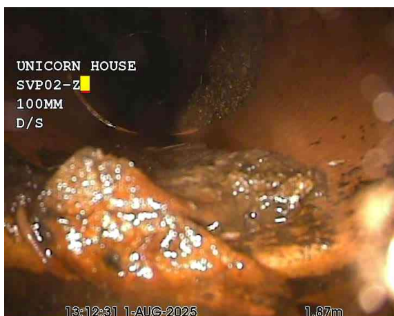
SVP02_f2d4391c-341d-4e74-bd4c-c5b495f712c8_20250807_121329_803.jpg, 00:00:29, 1.87 m Settled deposits, coarse at joint, 10% cross-sectional area loss
