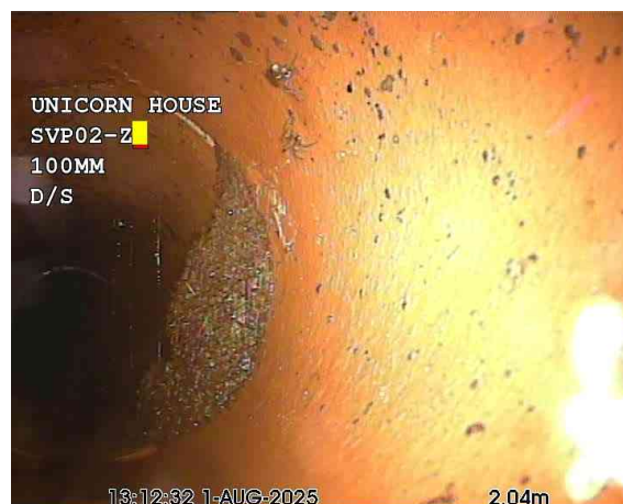
SVP02_14d57409-9fa7-4674-b56e-b180c7f38037_20250807_121408_857.jpg, 00:00:30, 2.04 m Roots, mass at joint, 20% cross-sectional area loss
