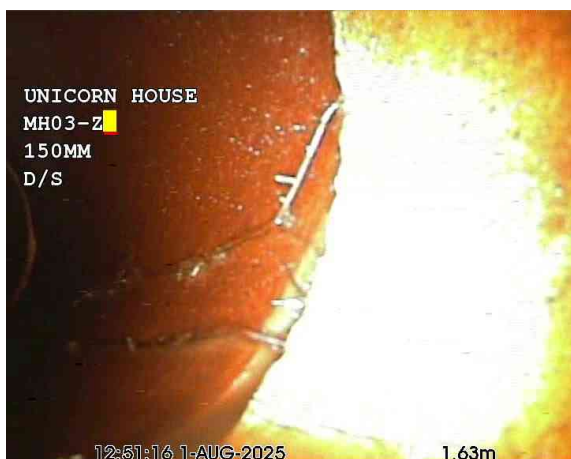
MH03_b0d99bc4-a16b-4ce5-9ed5-45eabae749cb_20250807_112326_449.jpg, 00:00:37, 1.63 m Roots, fine at joint
