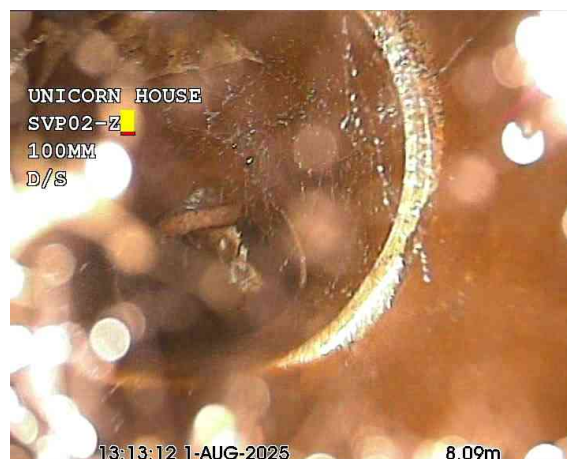
SVP02_8fbf373b-25dc-43e1-ae19-91f47e5ada06_20250807_121832_101.jpg, 00:01:10, 8.09 m Joint displaced, medium
