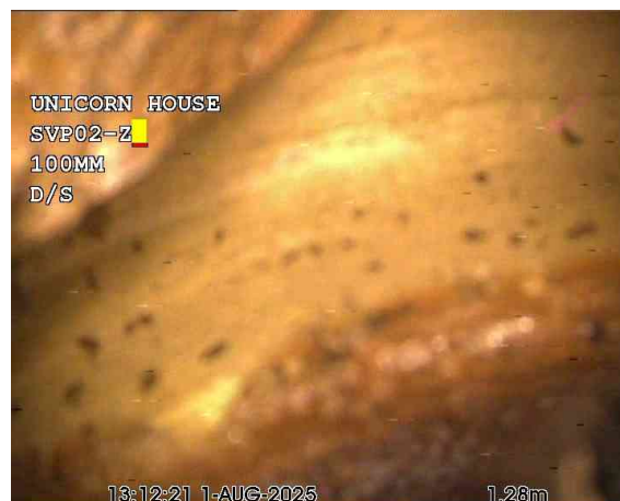
SVP02_2a13e2d1-06e3-4ebb-b9e0-a79efd186f7c_20250807_121111_101.jpg, 00:00:19, 1.28 m Joint displaced, medium
