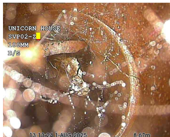
SVP02_e73e7fc4-fdc4-44e0-b572-71987eb8e0ba_20250811_100731_273.jpg, 00:01:22, 8.67 m Fracture, longitudinal at joint at 3 o'clock
