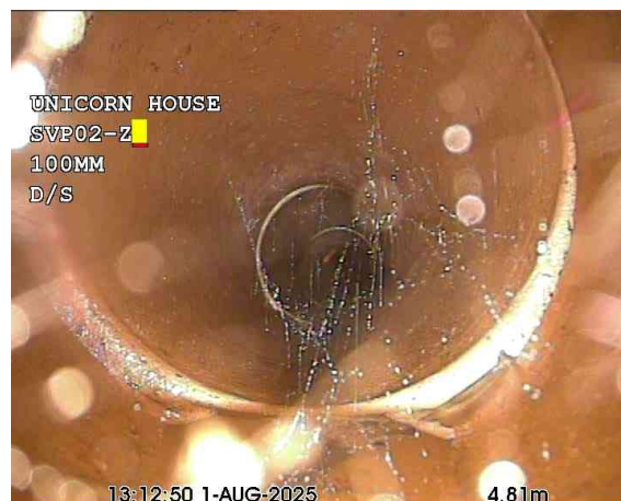
SVP02_09e43bbf-a4f6-45a7-a404-286cb7689d18_20250807_121559_550.jpg, 00:00:48, 4.81 m Joint displaced, medium
