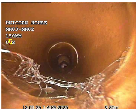
MH02_c4ef7829-8dec-489c-a4ef-74ee69762ce8_20250807_114844_710.jpg, 00:01:15, 9.80 m Roots, fine at joint
