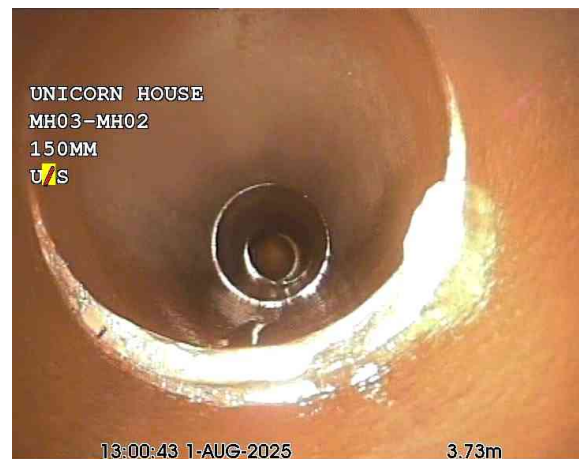
MH02_710311a1-3a8d-4aa4-b37d-ec0441cb5ca6_20250807_ 114201_976.jpg, 00:00:32, 3.73 m Joint displaced, large
