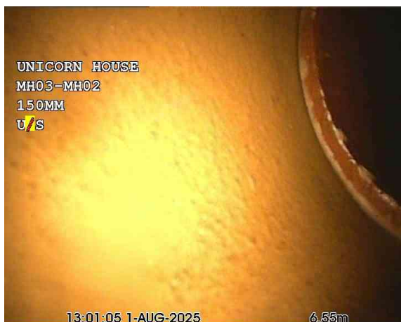
MH02_e23e6b2b-f858-4ab7-a288-551ee2282e7b_20250807_114632_938.jpg, 00:00:53, 6.55 m Joint displaced, medium
