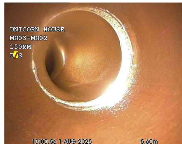
MH02_ff6dbb1e-2ff2-4a06-81ee-831824fb6ac6_20250807_114402_353.jpg, 00:00:45, 5.60 m Joint displaced, large
