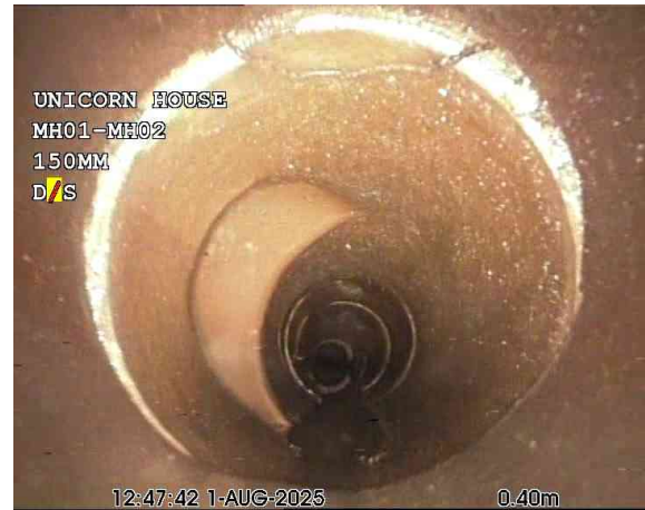
MH01_ded3a96f-066d-420b-a1dc-014538a649b7_20250807_ 110825_143.jpg, 00:00:07, 0.40 m Fracture, circumferential at joint from 11 o'clock to 1 o'clock
