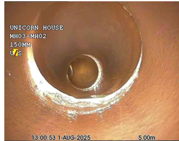
MH02_02d35aeb-b62b-454f-8103-db89c9ffc77f_20250807_114302_695.jpg, 00:00:42, 5.00 m Joint displaced, large
