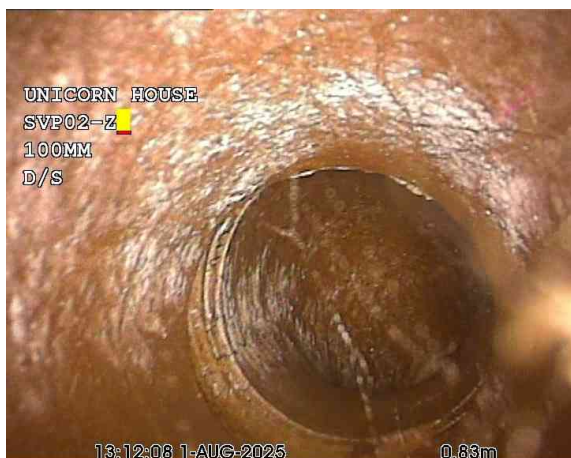
SVP02_044f1aeb-06de-45e9-8970-eb6db91e4d5_20250807_121000_519.jpg, 00:00:06, 0.83 m Joint displaced, large
