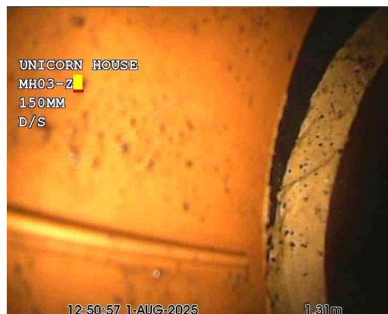
MH03_489e6729-736f-450f-9333-f8854997553f_20250807_112126_776.jpg, 00:00:18, 1.31 m Joint displaced, large
