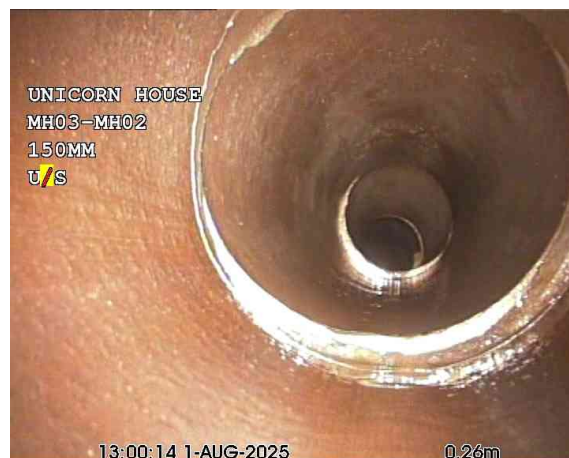
MH02_2d4e8cce-47b7-4ff8-b2a4-15a5cfe6edd2_20250807_1 13308_374.jpg, 00:00:03, 0.26 m Joint displaced, large
