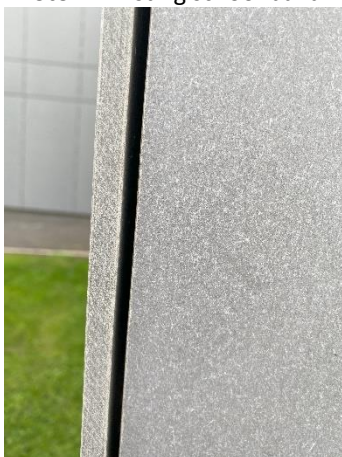
Photo 9: Gap between panels at existing school building
