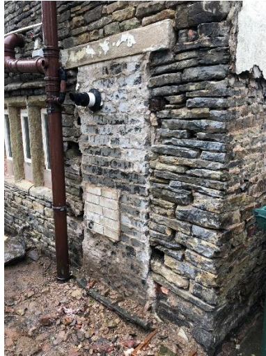
Picture 4. Image of part of the rear elevation with render removed showing an opening blocked with blue engineering brick.
