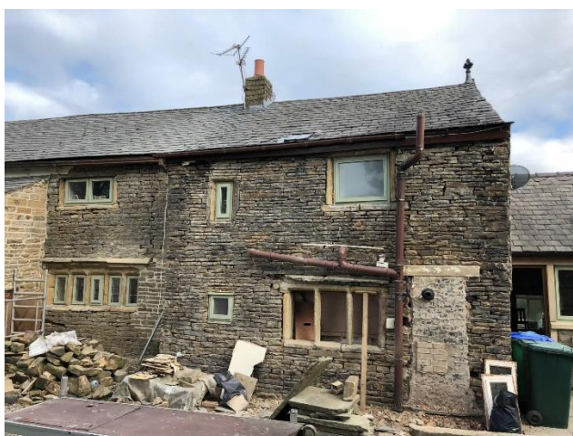
Picture 2. Image of part of the rear elevation with render removed.
