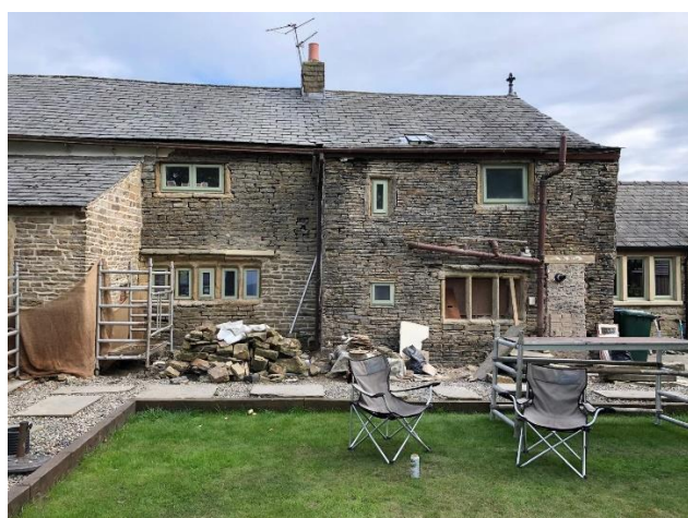
Picture 3. Image of part of the rear elevation with render removed.
