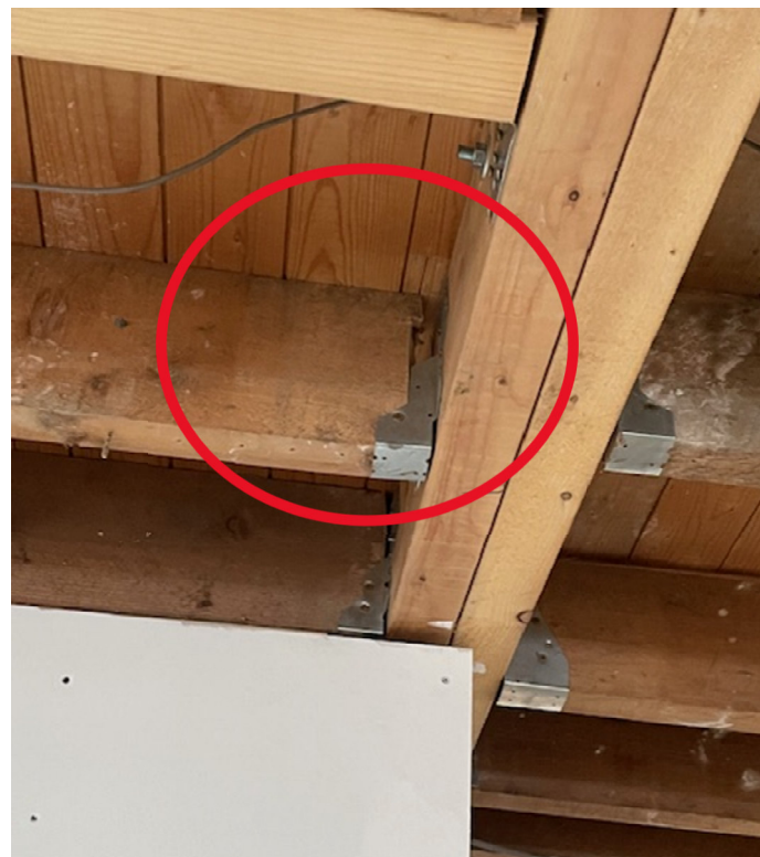
Photos showing typical incompliance of bearing of timber floor joints.
