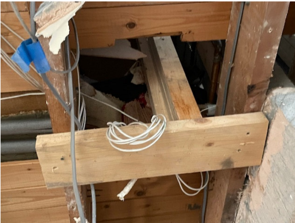
Photos showing incompliance detail of Timber Post Propping a Roof Purlin Supporting on a slender transfer timber member which fixed with a screw each end onto floor joists.
