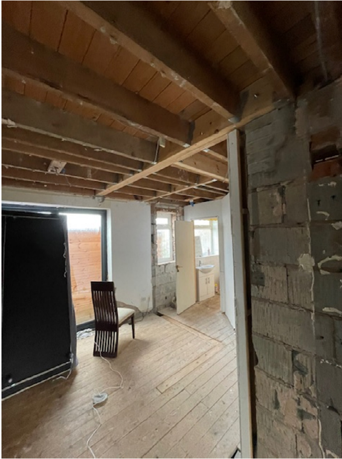
Photo Showing Dining Room with a Toilet – No Visible/Allowance for Shower/Bathroom.
