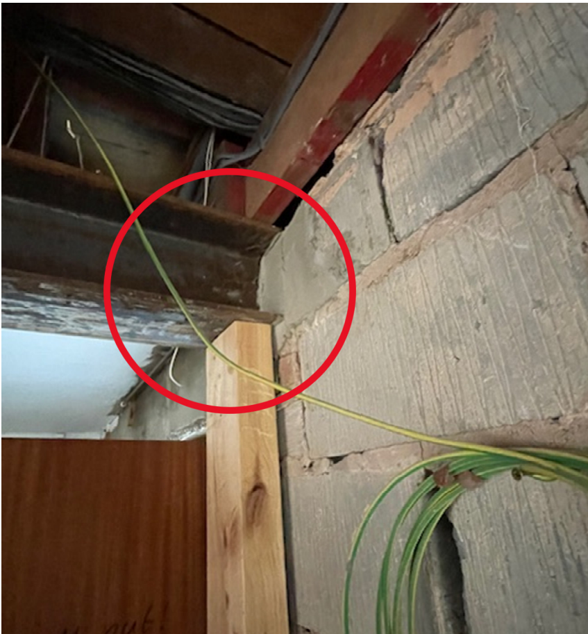
Incompliance transfer steel beam end supported on timber packing and a free standing timber post.
