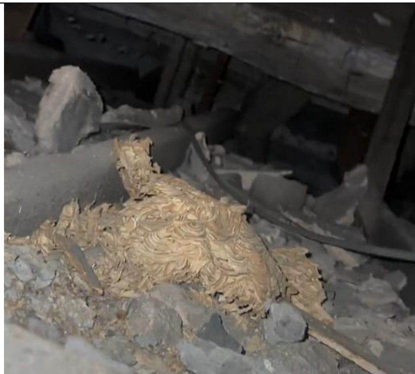
B1 Loft: Hornet's nest located on loft floor.
