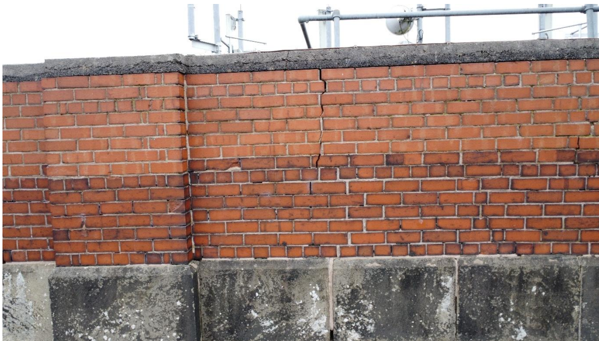
Photograph 1- Example of brickwork gap
