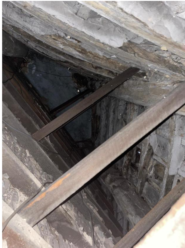
Figure 4: Deteriorated, sagging roof structure
