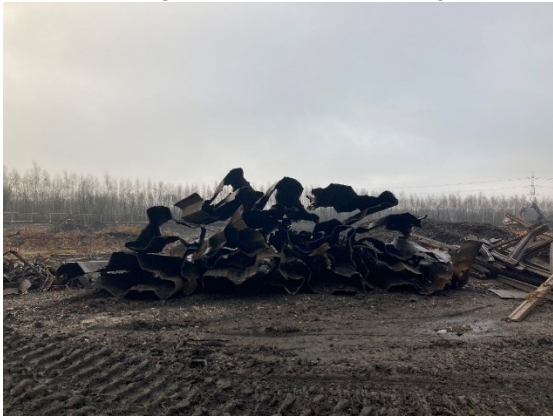
Plate 27 Scrap Metal For Off Site Disposal
