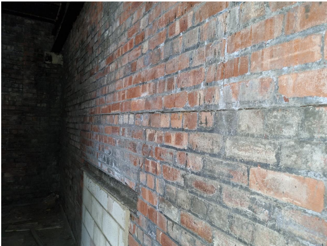
Corroded Embedded Steel within Bed Joints
