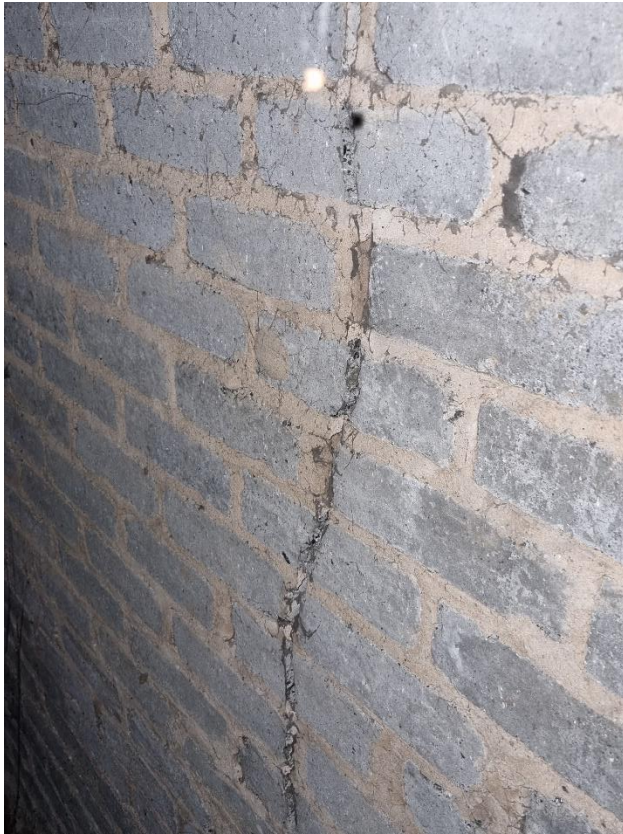
Cracking below Roof Beam
