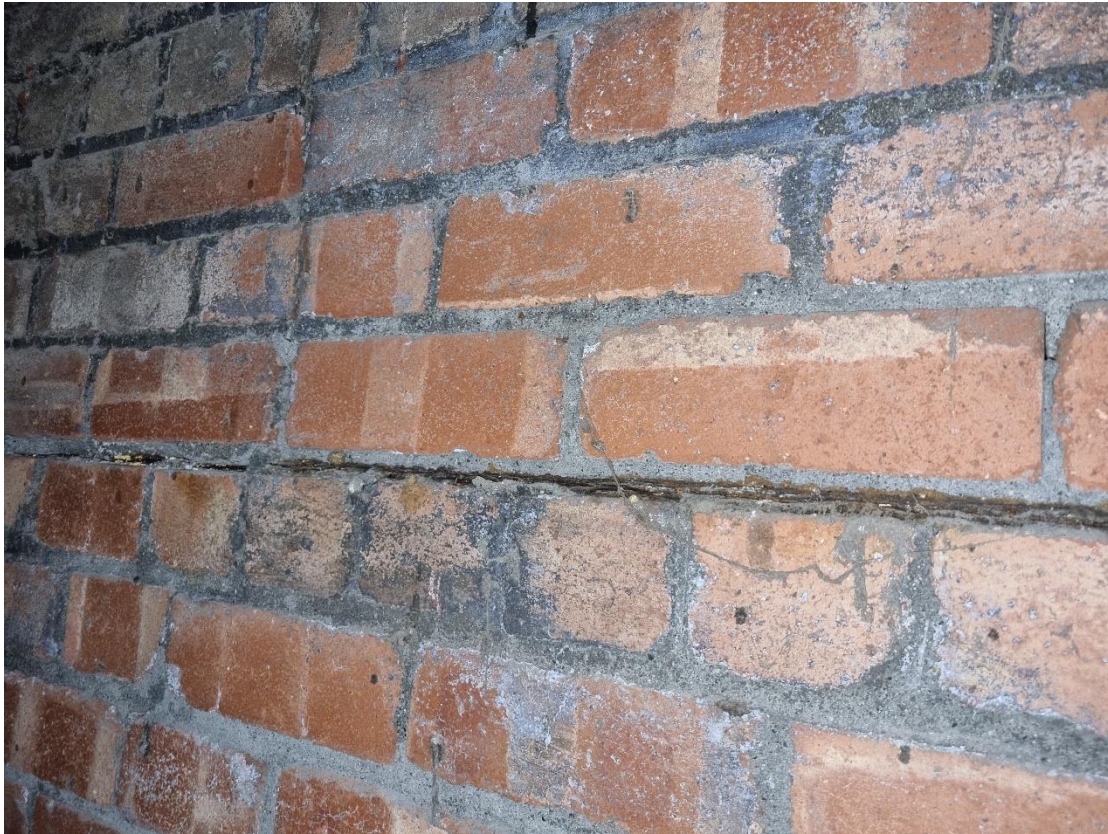
Corroded Embedded Steel within Bed Joints
