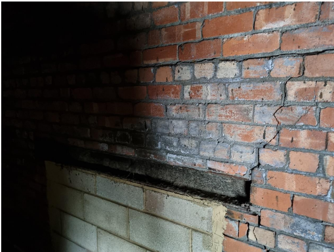
Corroded Steel Beam/Lintel
