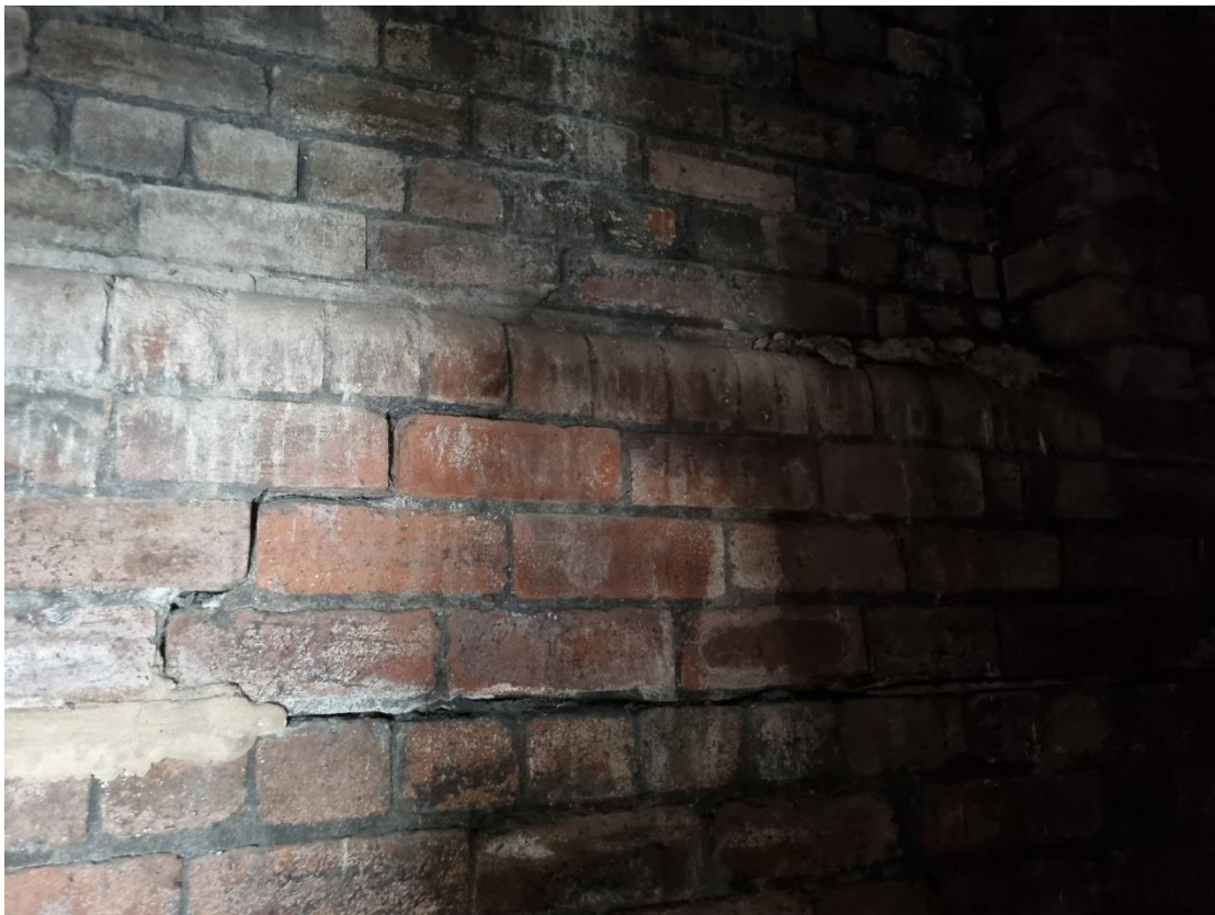
Cracking from Corroded Embedded Steelwork
