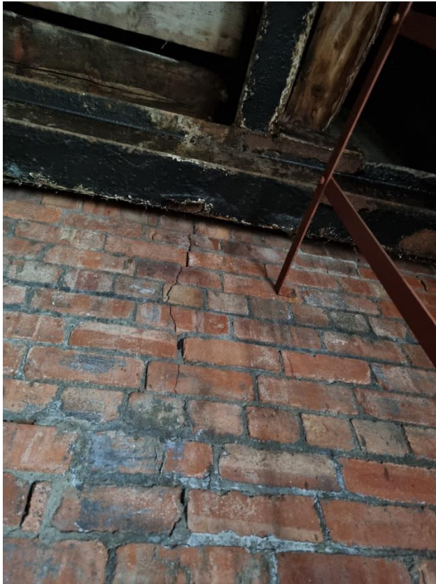
Cracking from Corroded Embedded Steelwork
