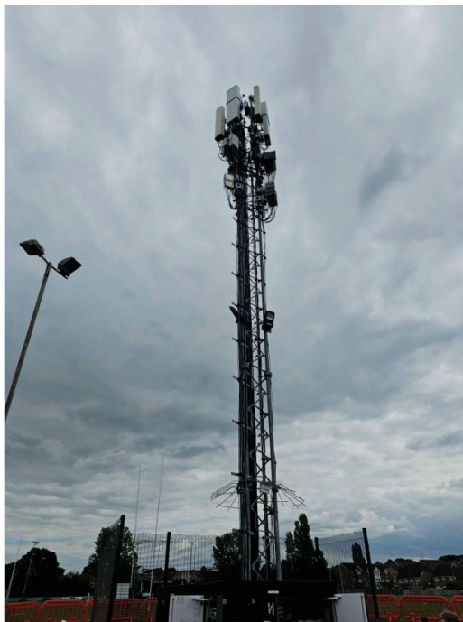
Image 2: Photo of lattice tower supporting antennas located at Sidcup Sports Ground
