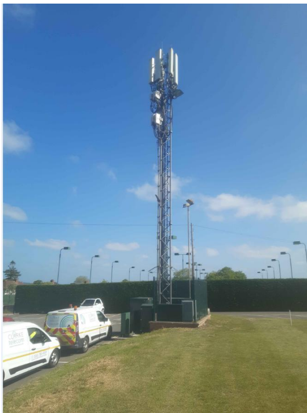
Image 3: Photo of lattice tower supporting antennas located at Sidcup Sports Ground
