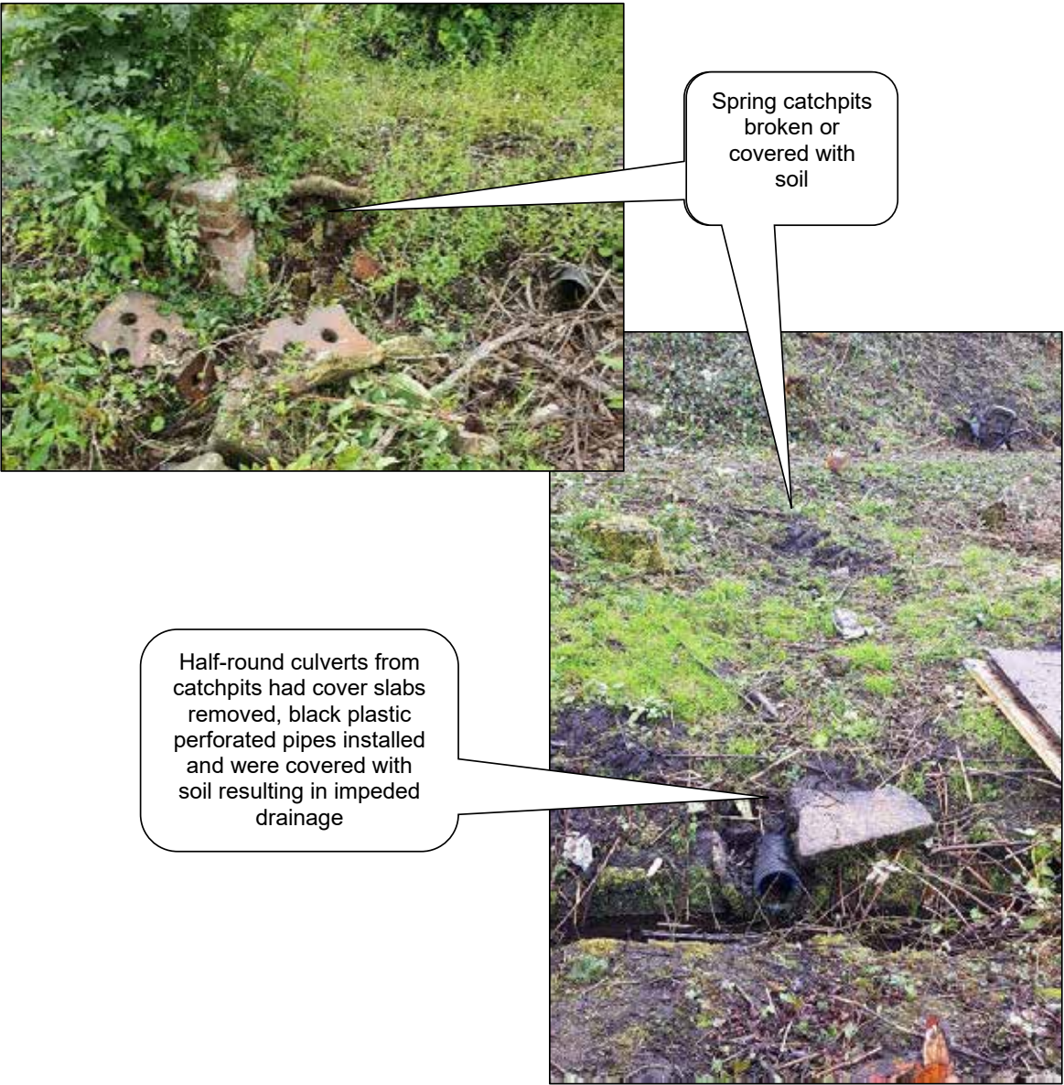
Figure 6.4 Packer Spout Top Spring Line Catchpits Broken or Covered With Soil – Half-Round Culverts from Catchpits Have Cover Slabs Removed, Black Plastic Perforated Pipes installed and Are Covered with Soil Resulting In Impeded Drainage
