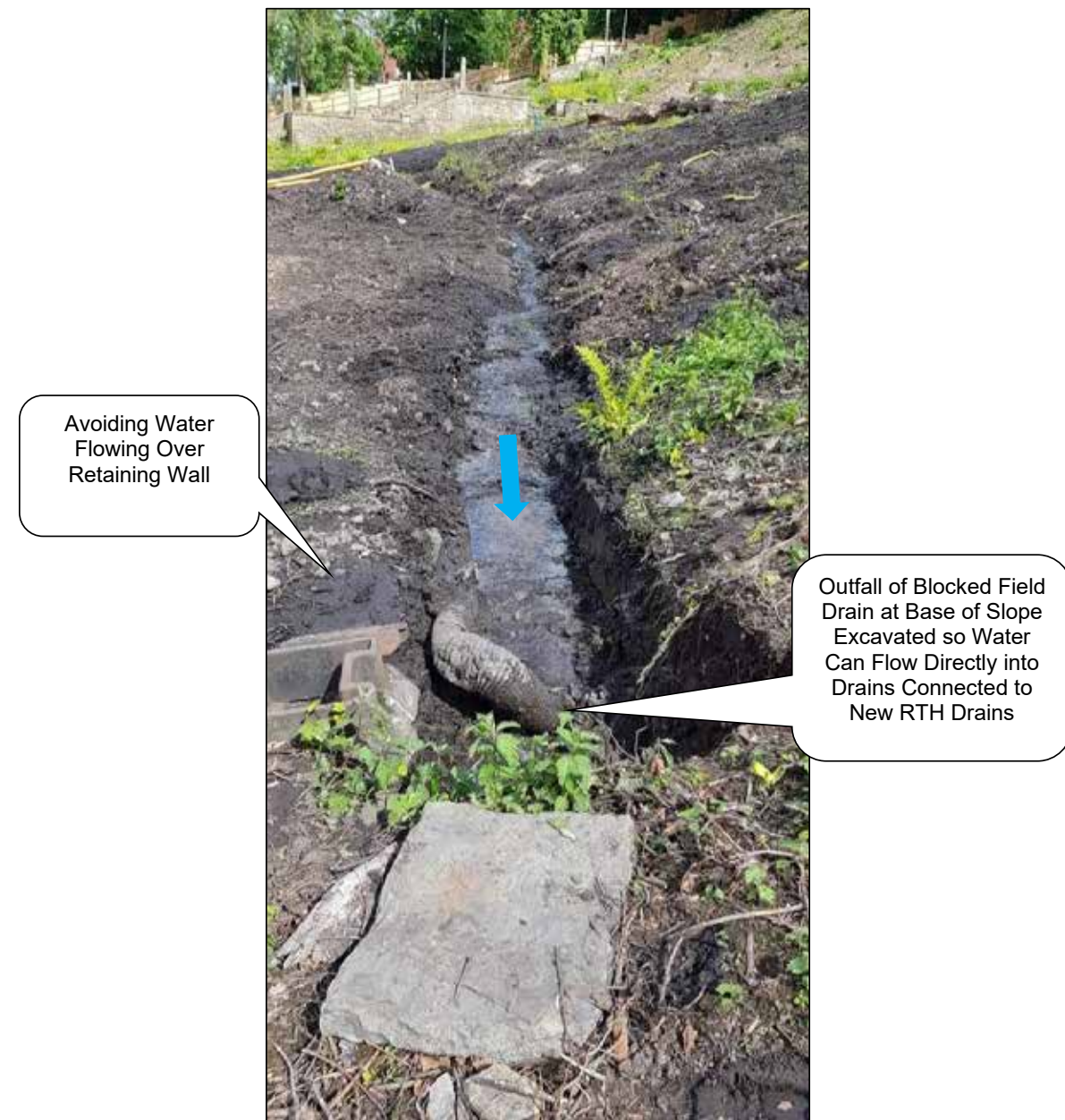
Fig. 8.1 Outfall of Blocked Field Drain at Base of Slope Excavated so Water Can Flow Directly into Drains Connected to New RTH Drains – Avoiding Water Flowing Over Retaining Wall
