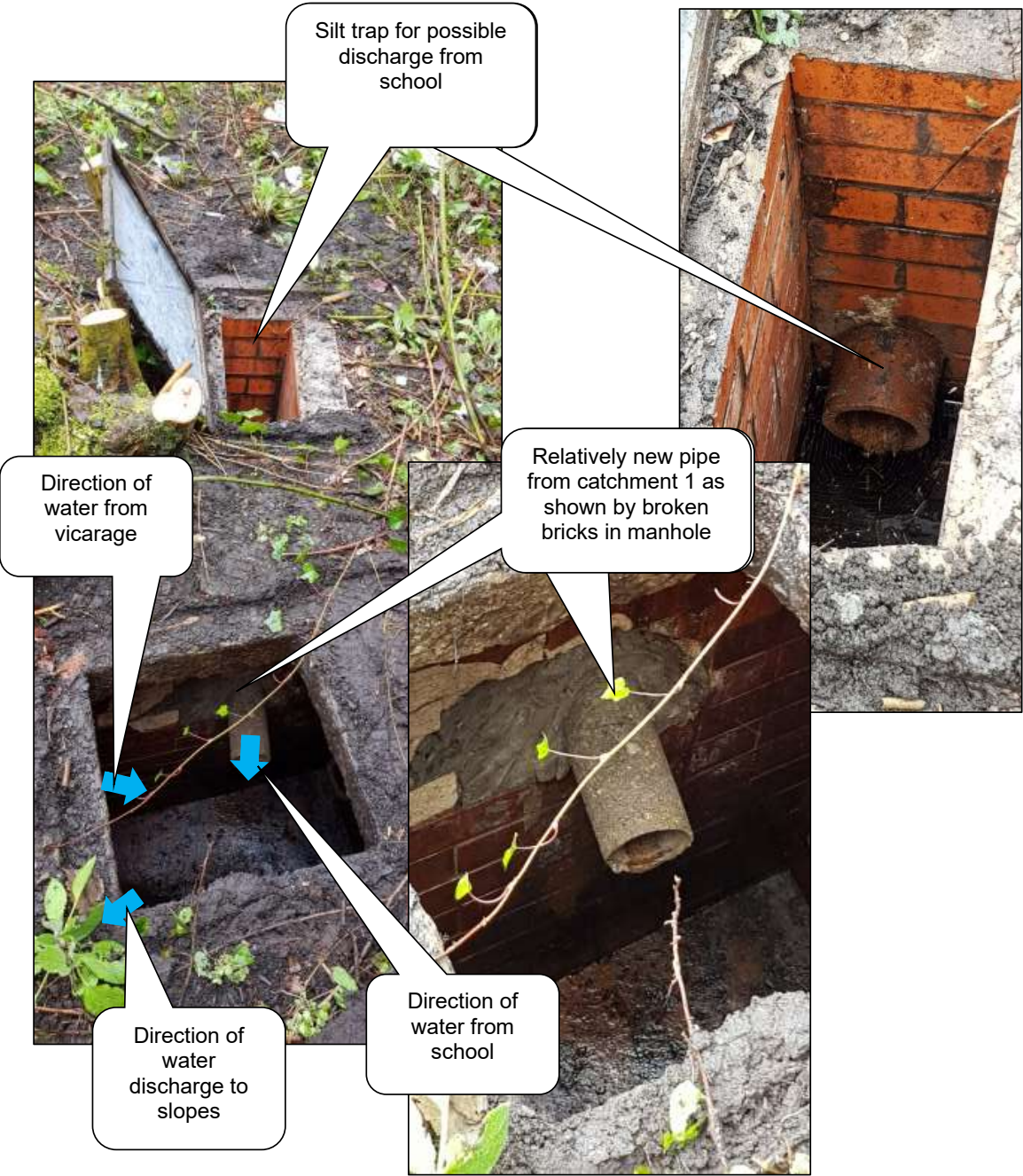
Manhole Next to Garden Gate Receiving Runoff from Catchment 1 (School playing fields) and Catchment 2 (Vicarage) and then Discharging to the Slopes
