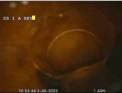
Photo: 5_7a, 00:00:00 1.5m, Joint displaced. Large
