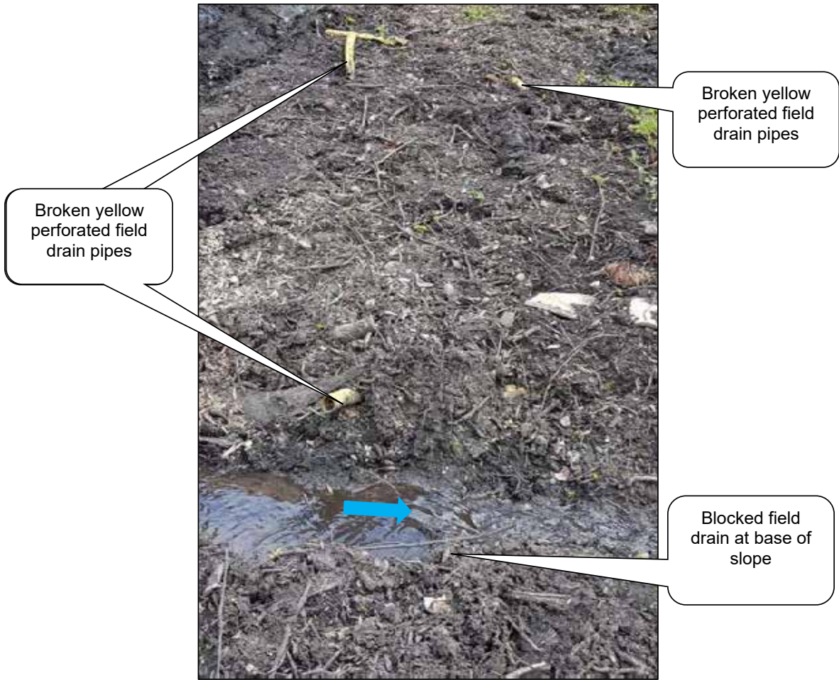
Fig. 7.2 Broken Yellow Field Drain Pipes above Field Drain at Base of Slope
