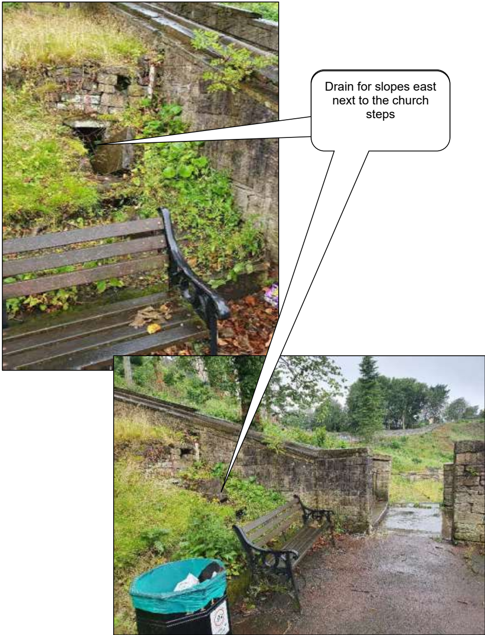
Fig. 16.2 Significant Drain for Catchment 6 – Slopes East Next to Church Steps
