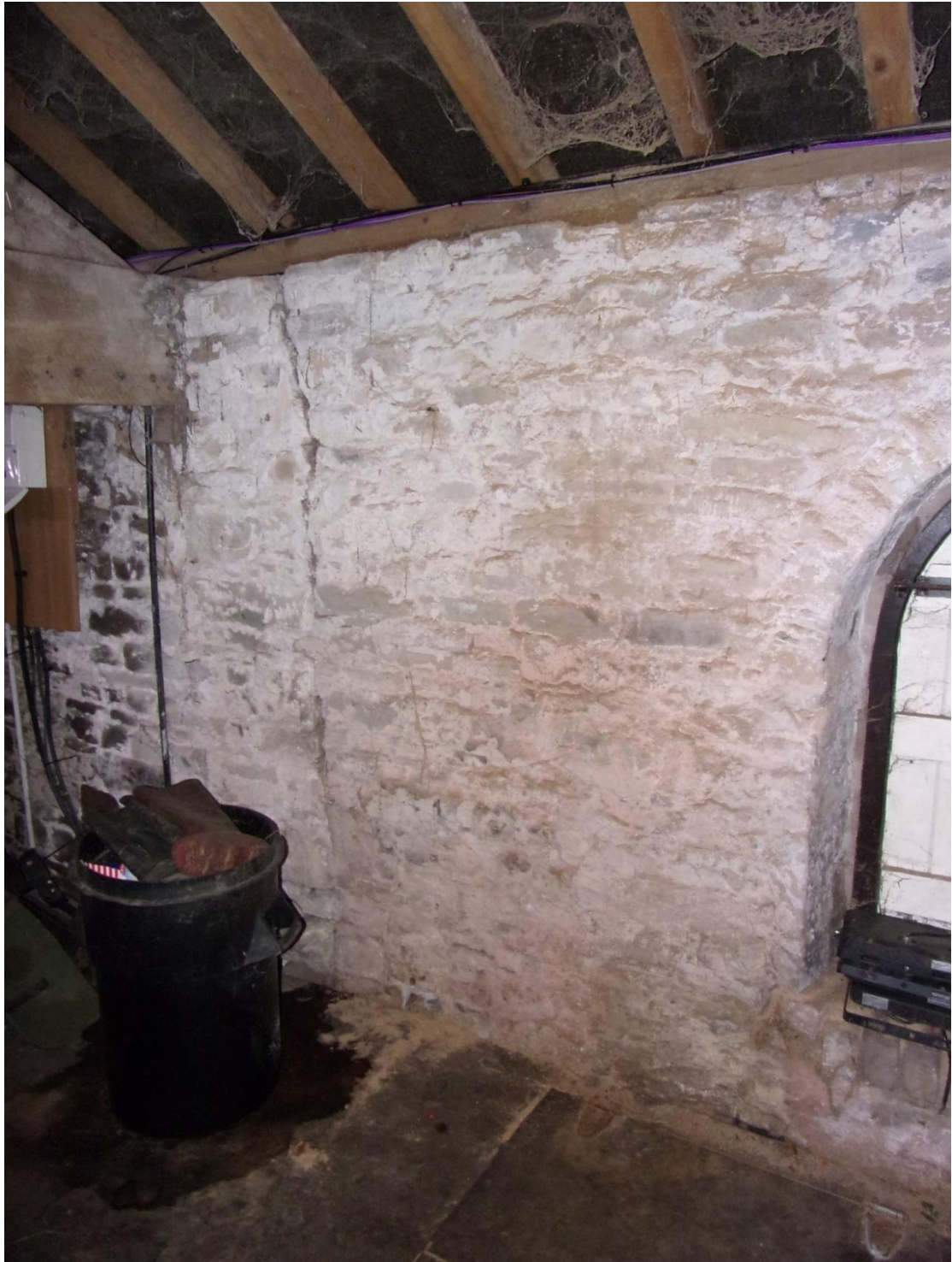
Plate 68 Wall crack in the south elevation of Room 13
