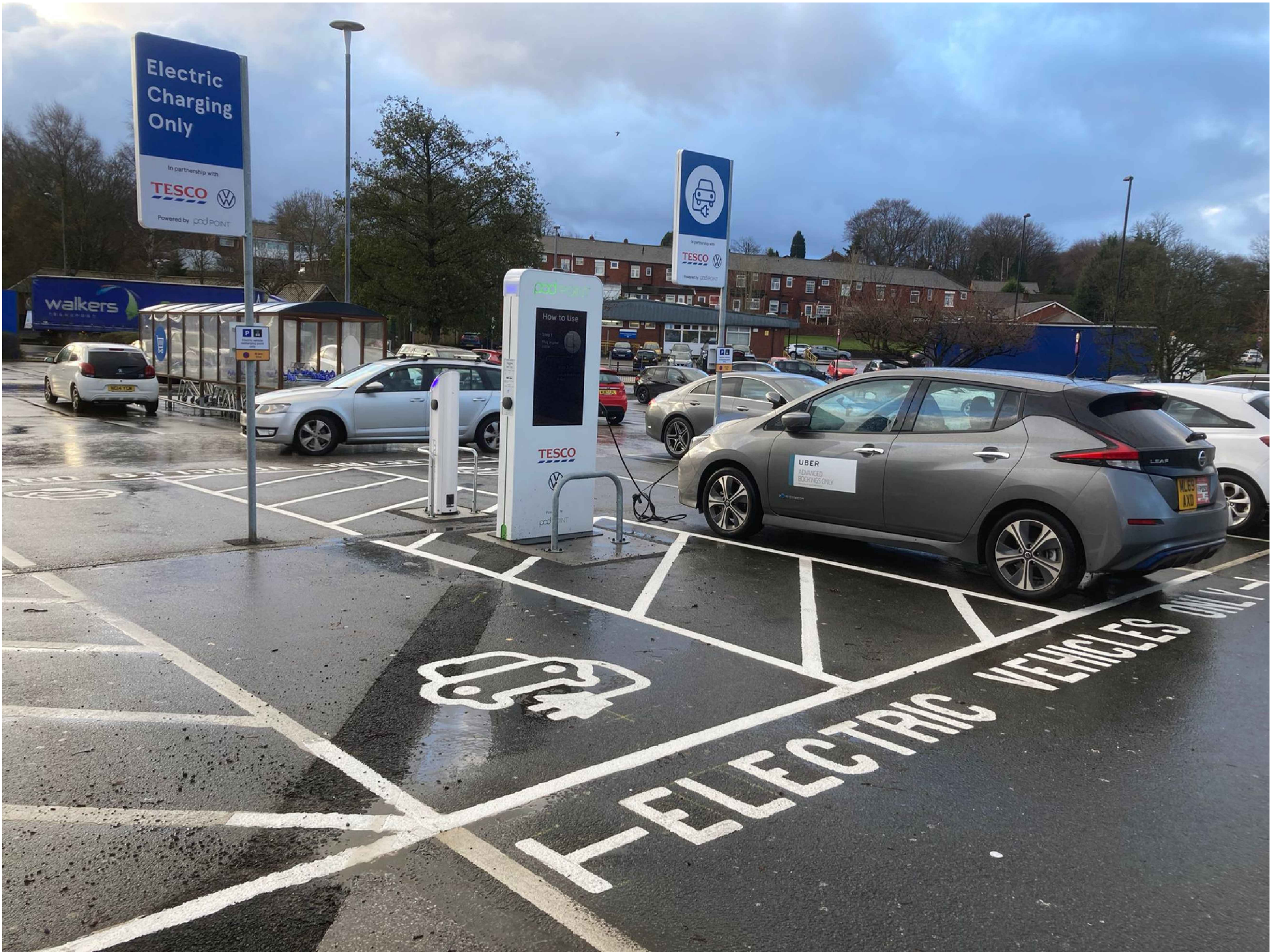
ELECTRIC VEHICLE-CHARGING AREA AT SITE
