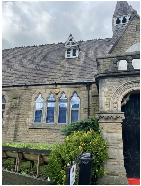
Ridge Tiles damaged near Cupola
