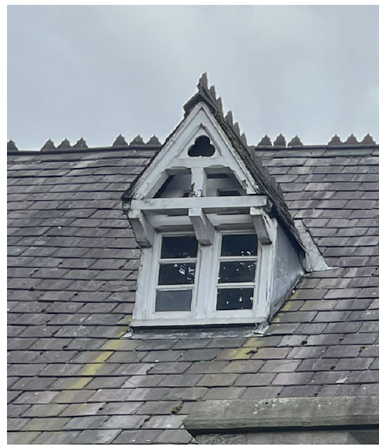
C3 Dormer woodwork damaged; requires further inspection
