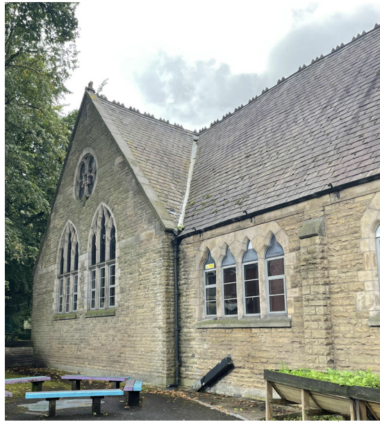
Multiple damaged Ridge Tiles
