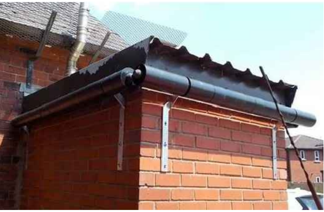
example of anti climb rollers
