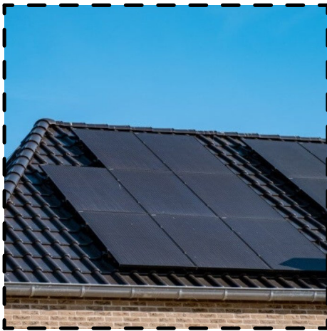
Solar Panels - External Roofs
