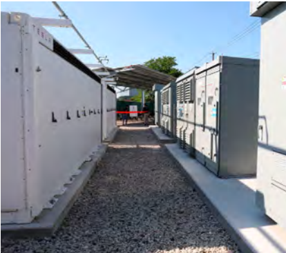
Battery storage units in greys
