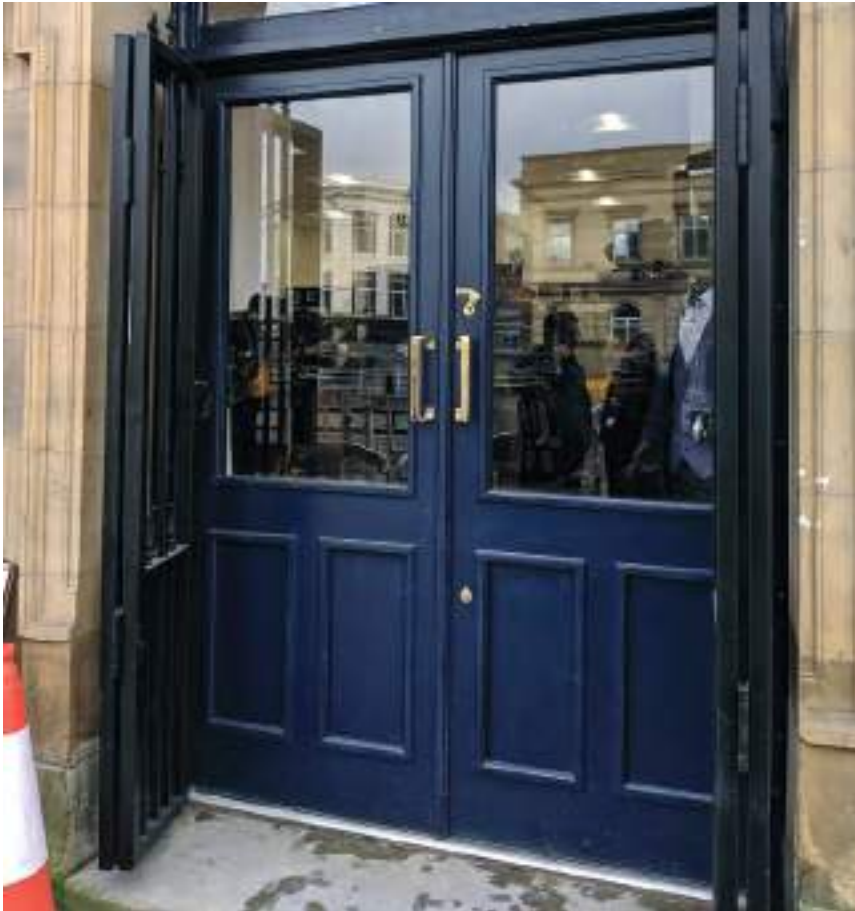
GOOD EXAMPLE OF EXTERNAL GATE TO DOORS
