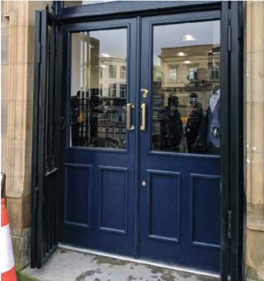
GOOD EXAMPLE OF EXTERNAL GATE TO DOORS
