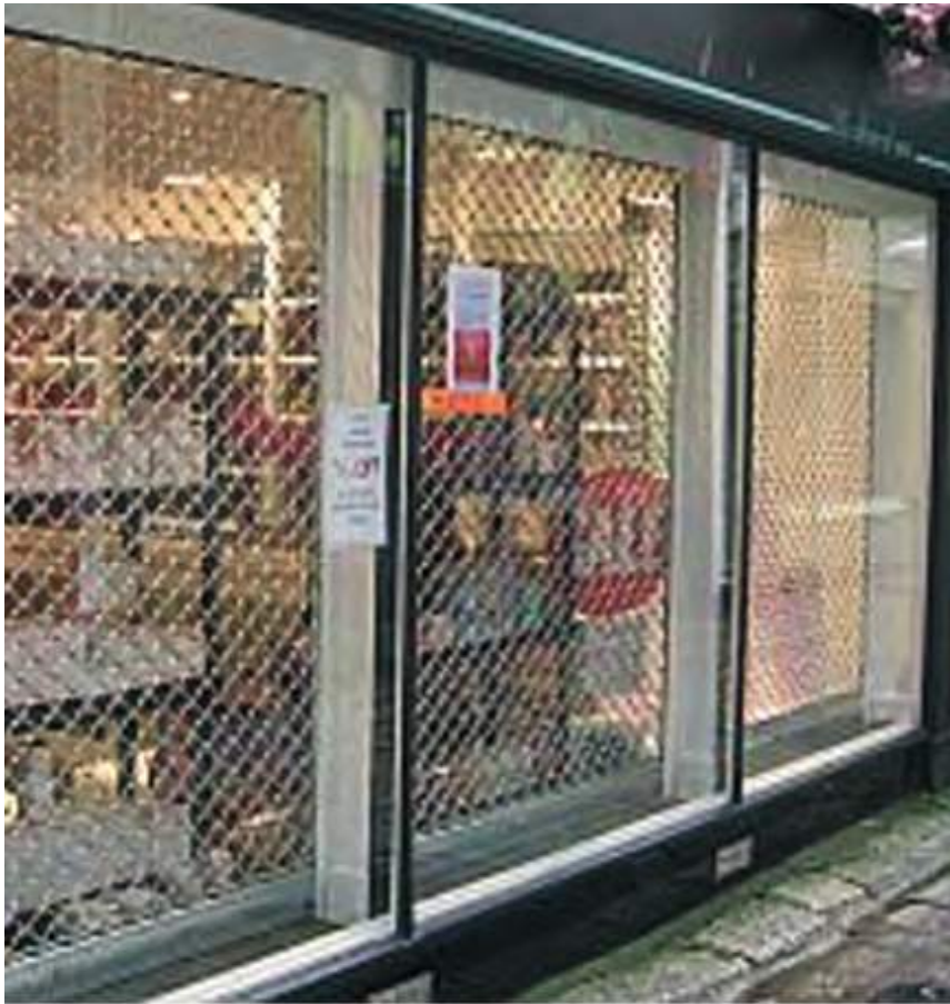
INTERNAL SECURITY GRILLES
