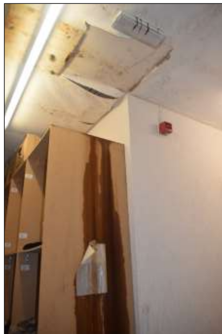
Photo 10: 18 Sadler Street - water ingress, first floor
