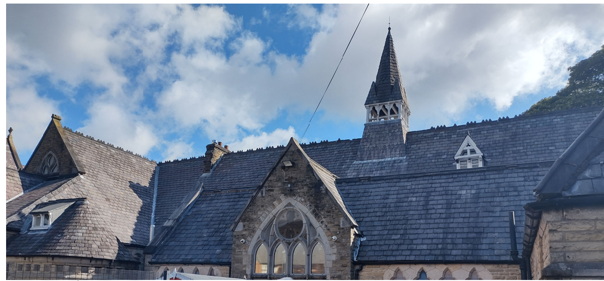
Broken Ridge Tiles mainly around Cupola
