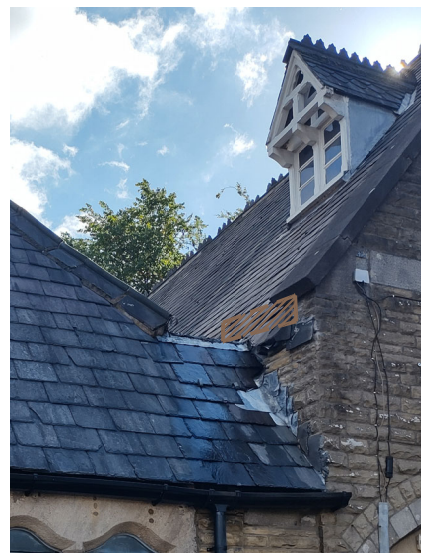
Additional guttering required in this area
