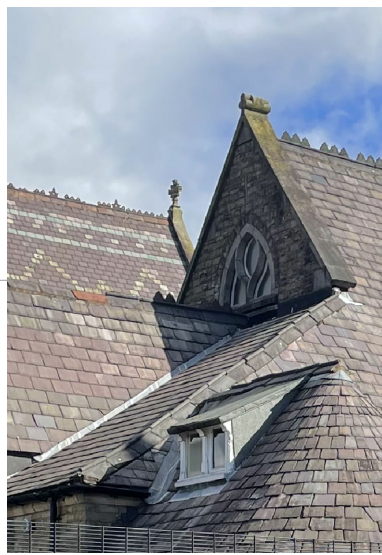
Significant Ridge tile damage in this area
