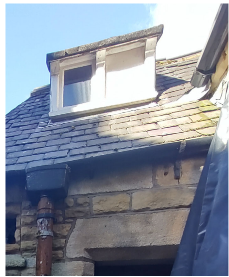
G1 Non-Gabled 'Shed' Dormer Windows require re-felting
