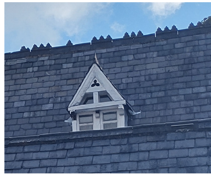
C4 Dormer window woodwork requires repainting
