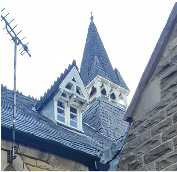
C3 Dormer window woodwork requires repainting
