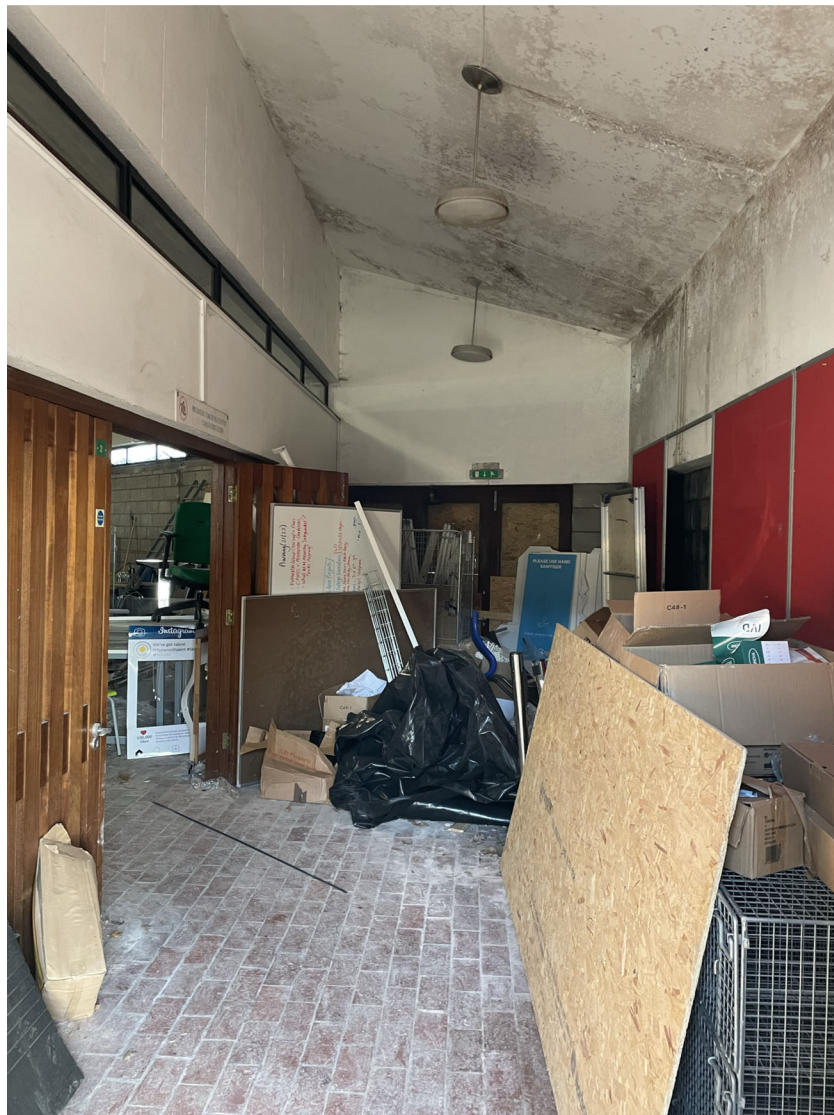
Interior View showing water damaged Narthex ceiling to be removed
