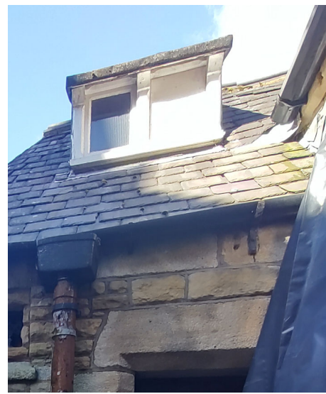
G1 Non-Gabled 'Shed' Dormer Windows require re-felting
