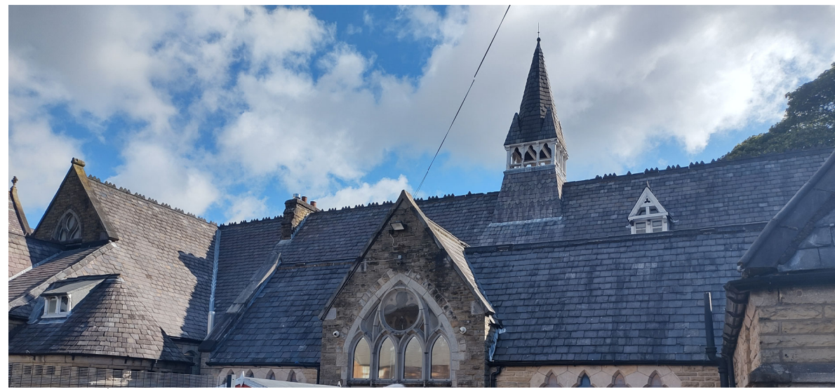
Broken Ridge Tiles mainly around Cupola
