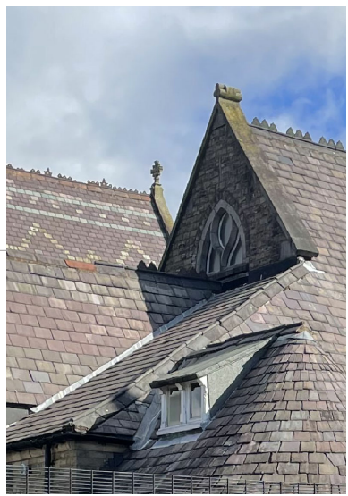
Significant Ridge tile damage in this area
