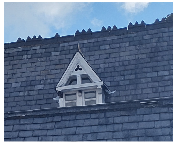
C4 Dormer window woodwork requires repainting
