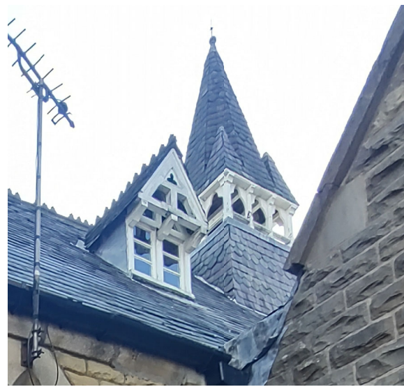
C3 Dormer window woodwork requires repainting
