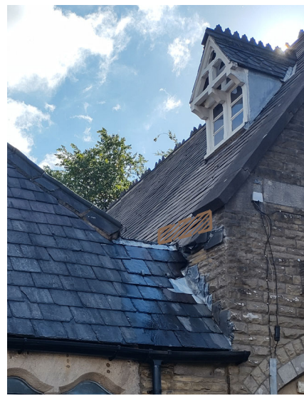
Additional guttering required in this area
