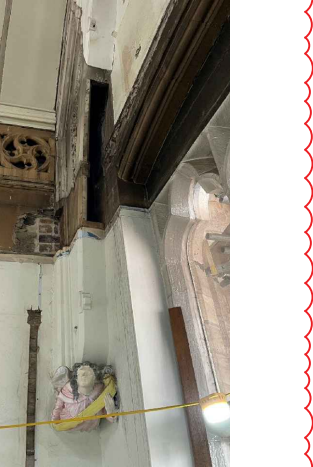
IMAGE 6 - Gap in truss, hardboard to be put back.
