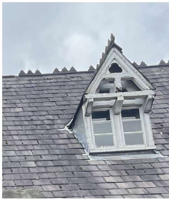
C4 Dormer wooden structure damaged; will require replacement sections
