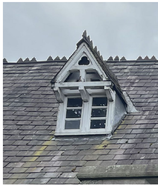
C3 Dormer wooden structure damaged; requires further inspection
