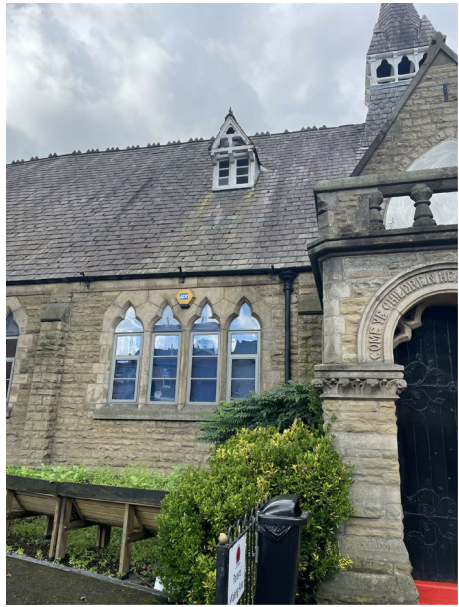
Ridge Tiles damaged near Cupola
