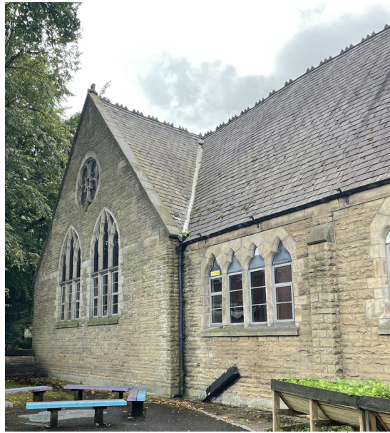
Multiple damaged Ridge Tiles
