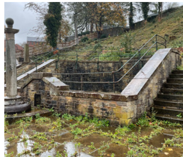
3.54 Packer Spout Fountain at the centre of the built feature
