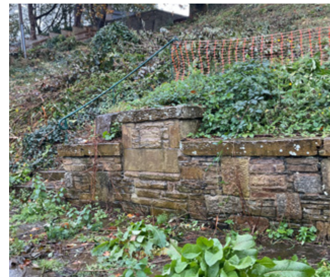
3.60 Possible lost plaque on the retaining wall to the gardens
