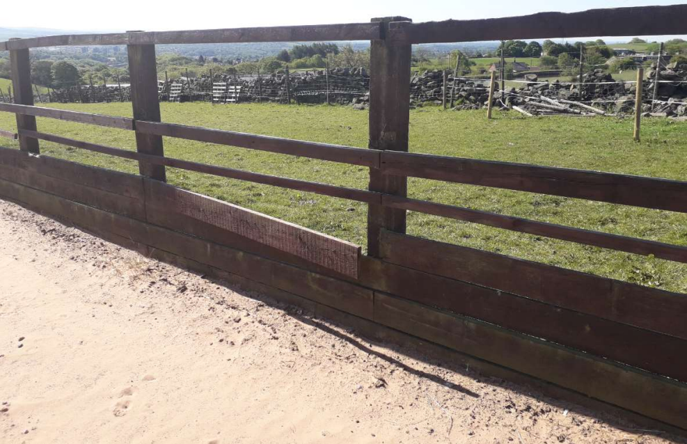
Pictures of condition of current arena:
