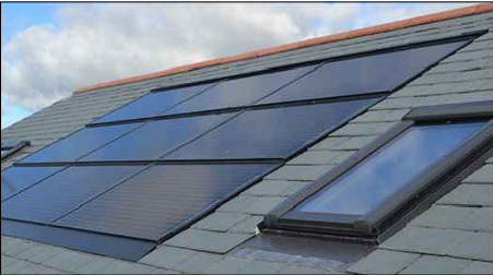
9. inset photovoltaic panels
