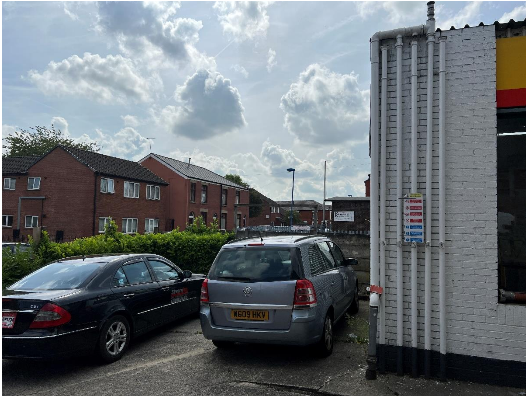
Existing Vent Stacks from Petrol Tanks
