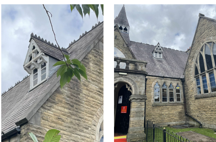
A2 Dormer wood paintwork worn; requires further inspection Downpipe rusted; requires sanding down & repainting
