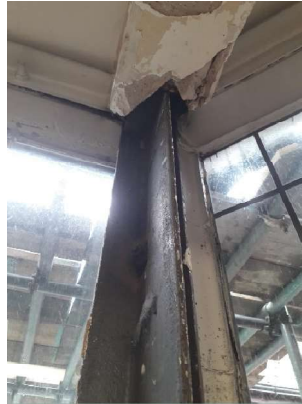
Vertical mullion support steel and corroding fixings into the stone
