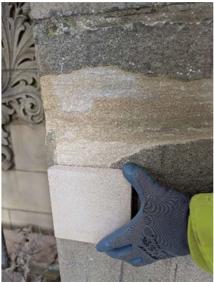
Loose/spalling stone facings removed and sample provided for stonework
