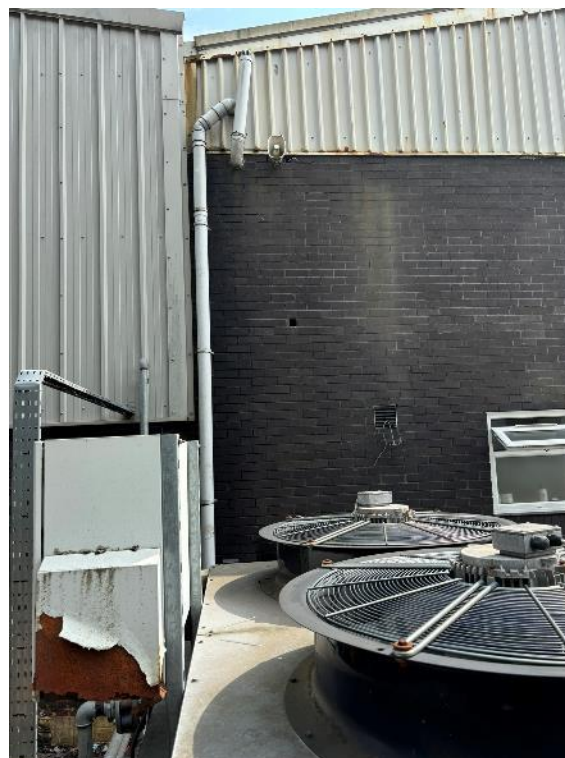
Photograph 4: Section of missing brick on west elevation. Not considered to be affected by proposals and within very noisy and heavily lit building. Negligible.
