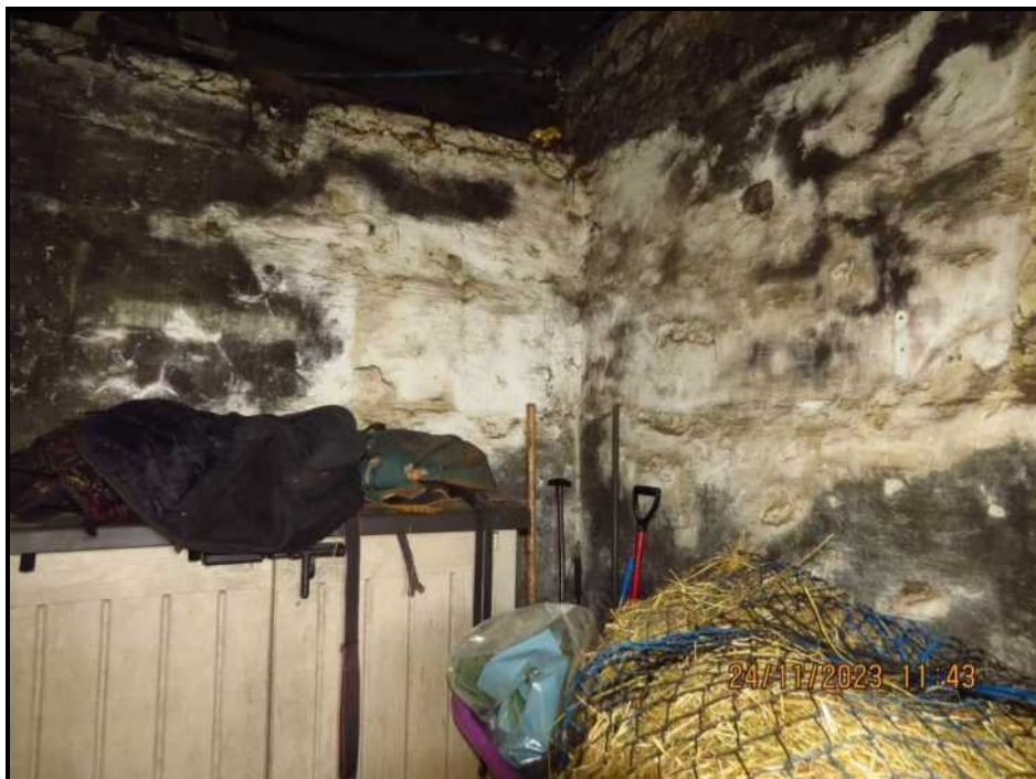
044 Lower wall, Northern corner
