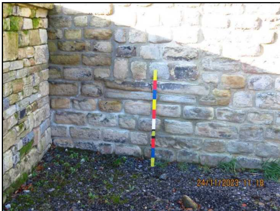
006 No signs of separation between wall structures
