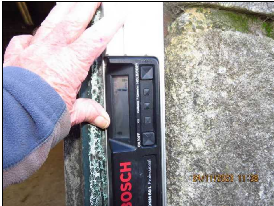
030 Good vertical alignment to right hand reveal
