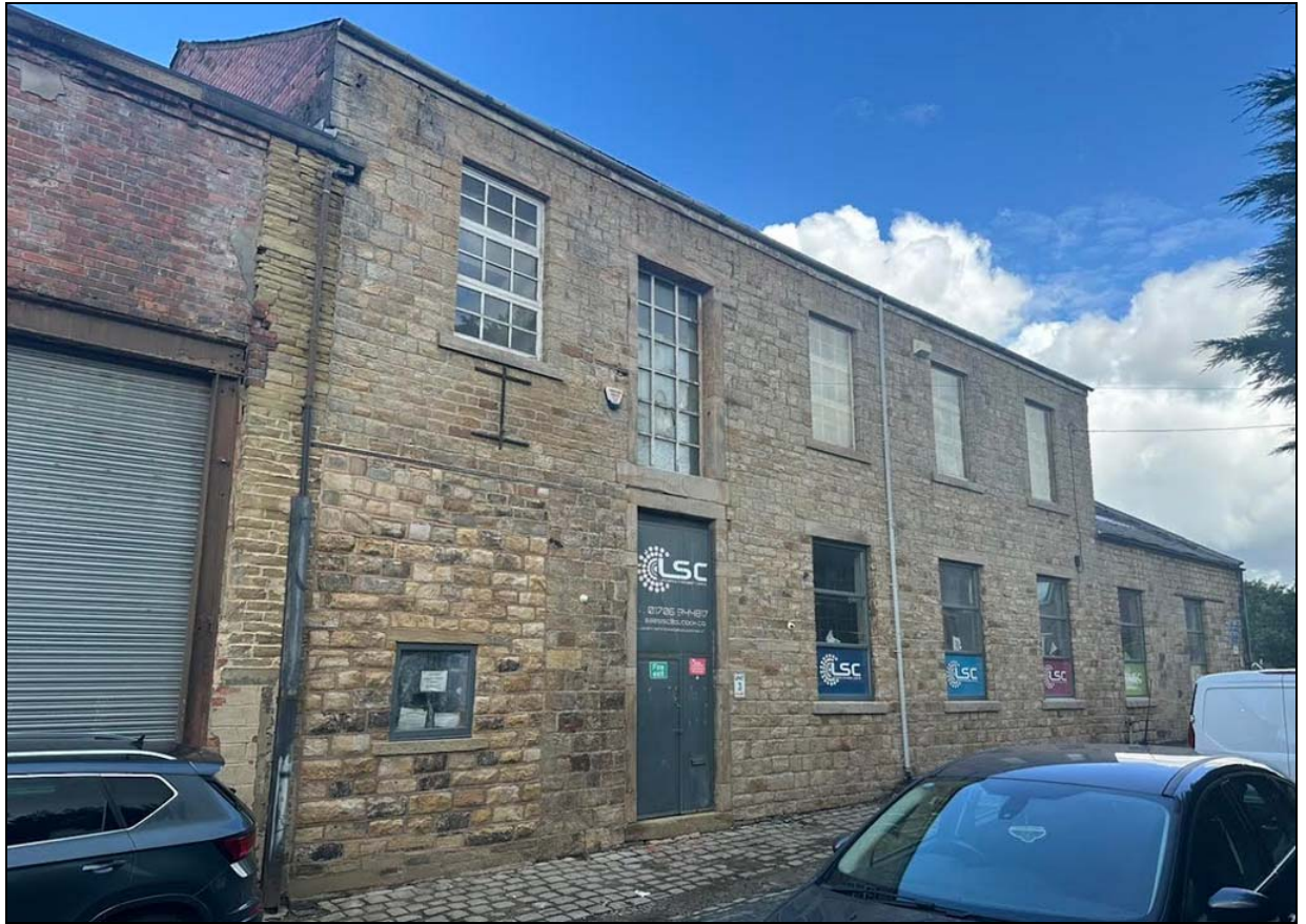
3. Front elevation: blocked loading bay door to left of entrance
