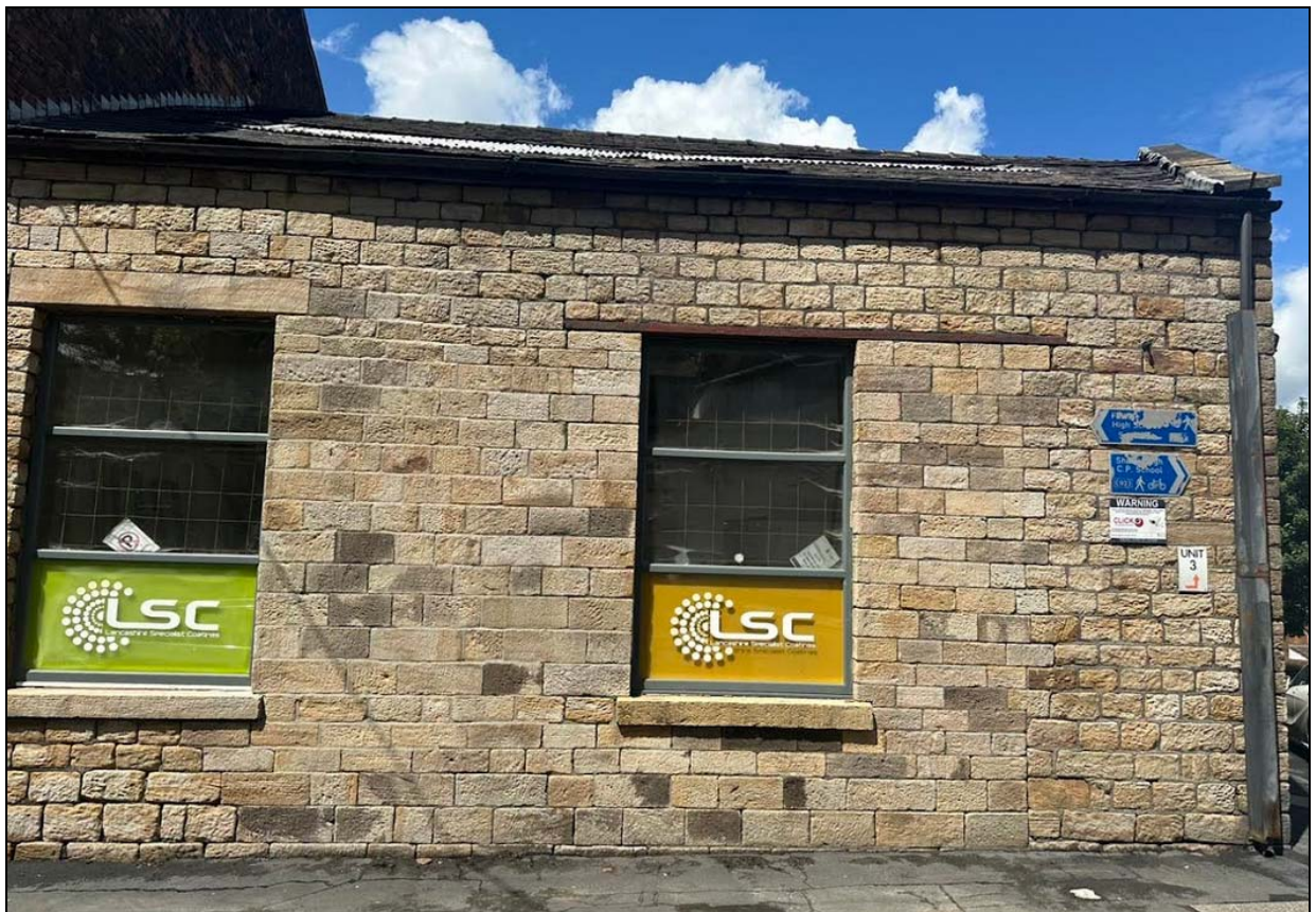
4. Evidence of another blocked loading door on right of the single-storey element
