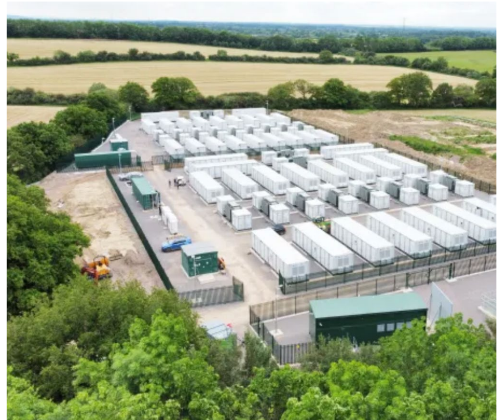
Minety BESS, Wiltshire - Penso Power
