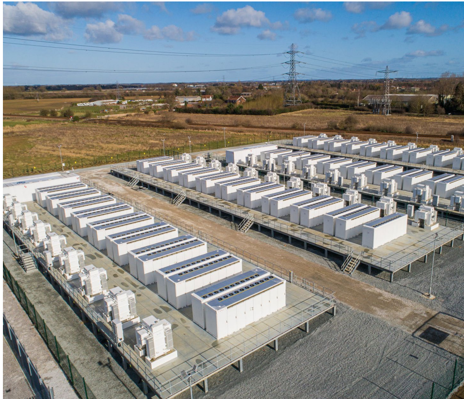
BESS, Pillswood - Harmony Energy
