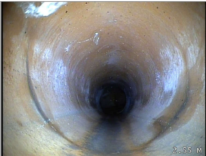
Crack circumferential from 2 to 10 o'clock
