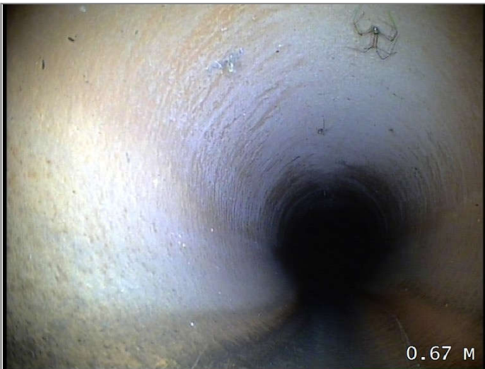
Fracture multiple from 7 to 1 o'clock, Finished
