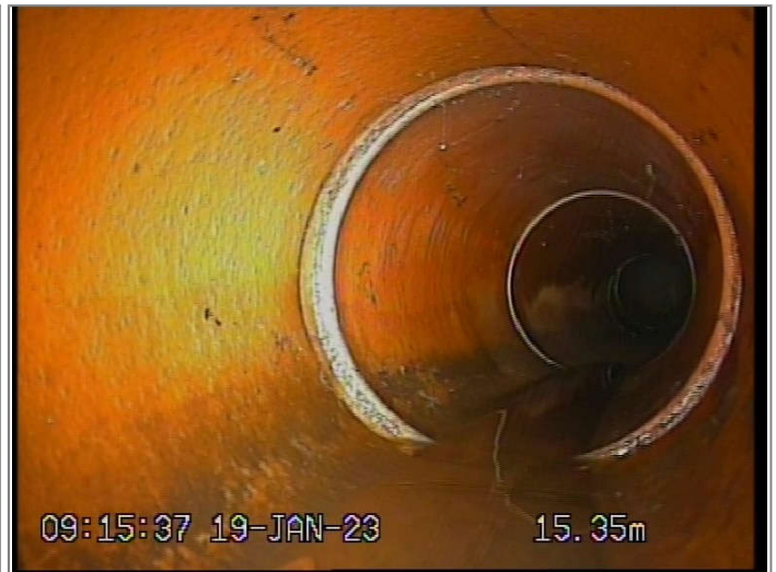
Line of drain/sewer deviates right
