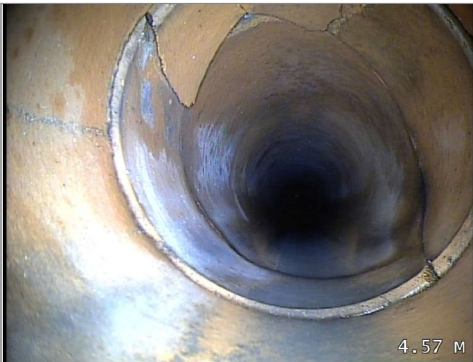
Fracture multiple from 10 to 5 o'clock
