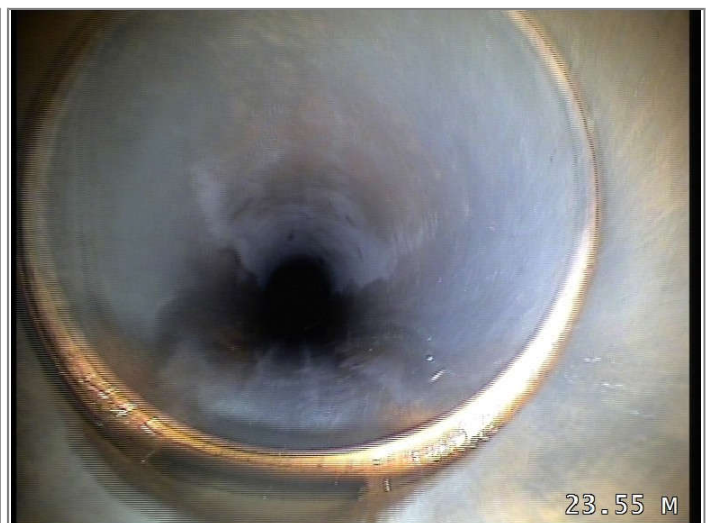
Joint displaced medium
