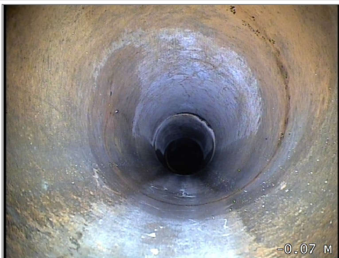
Crack circumferential from 1 to 10 o'clock
