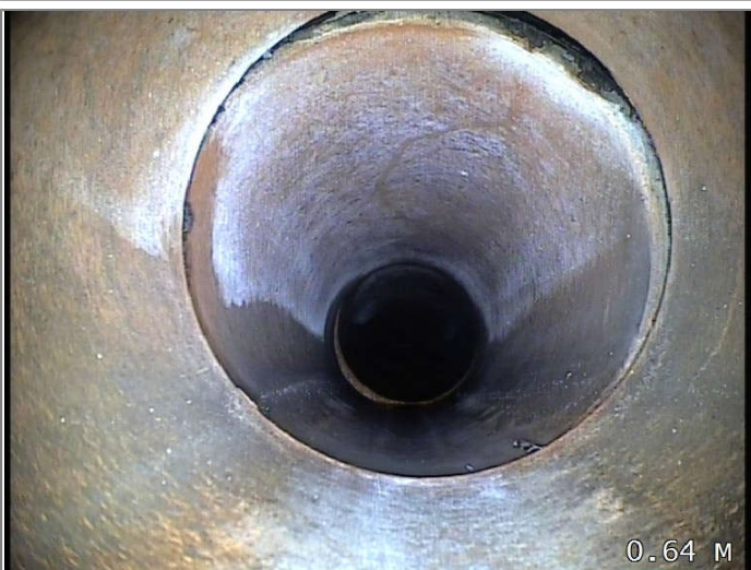
Joint displaced medium
