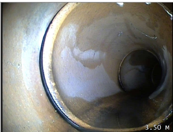
Line of drain/sewer deviates right
