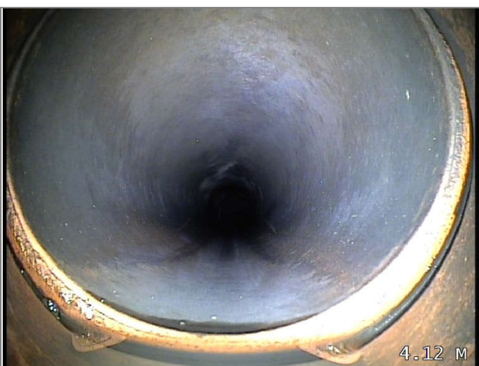
Joint displaced medium - Remark: SEAL VISABLE
