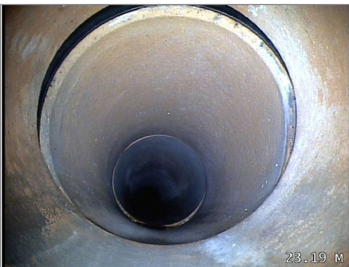
Joint displaced large
