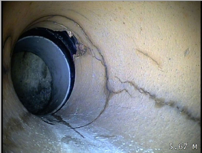
Line of drain/sewer deviates left
