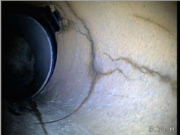
Fracture multiple from 12 to 12 o'clock
