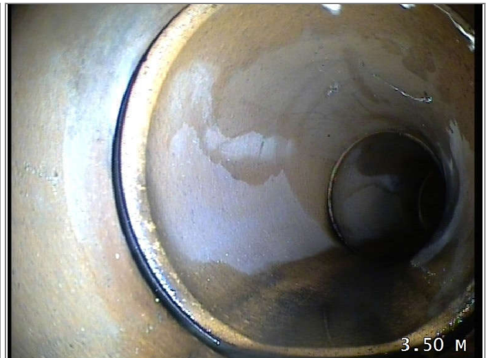
Joint displaced medium - Remark: SEAL VISABLE
