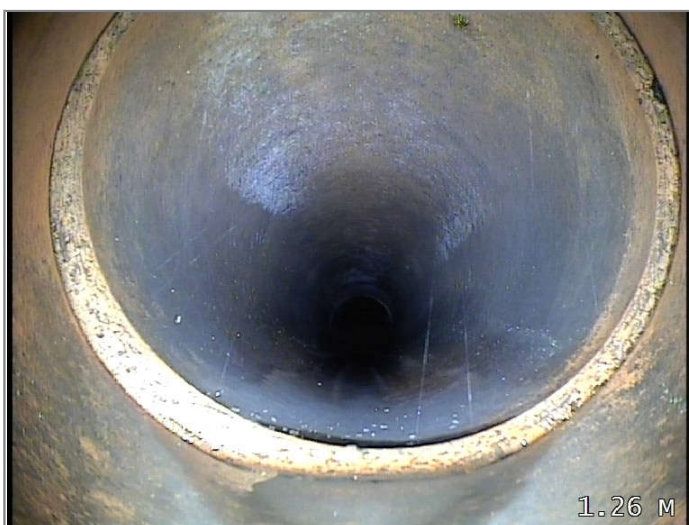
Joint displaced medium
