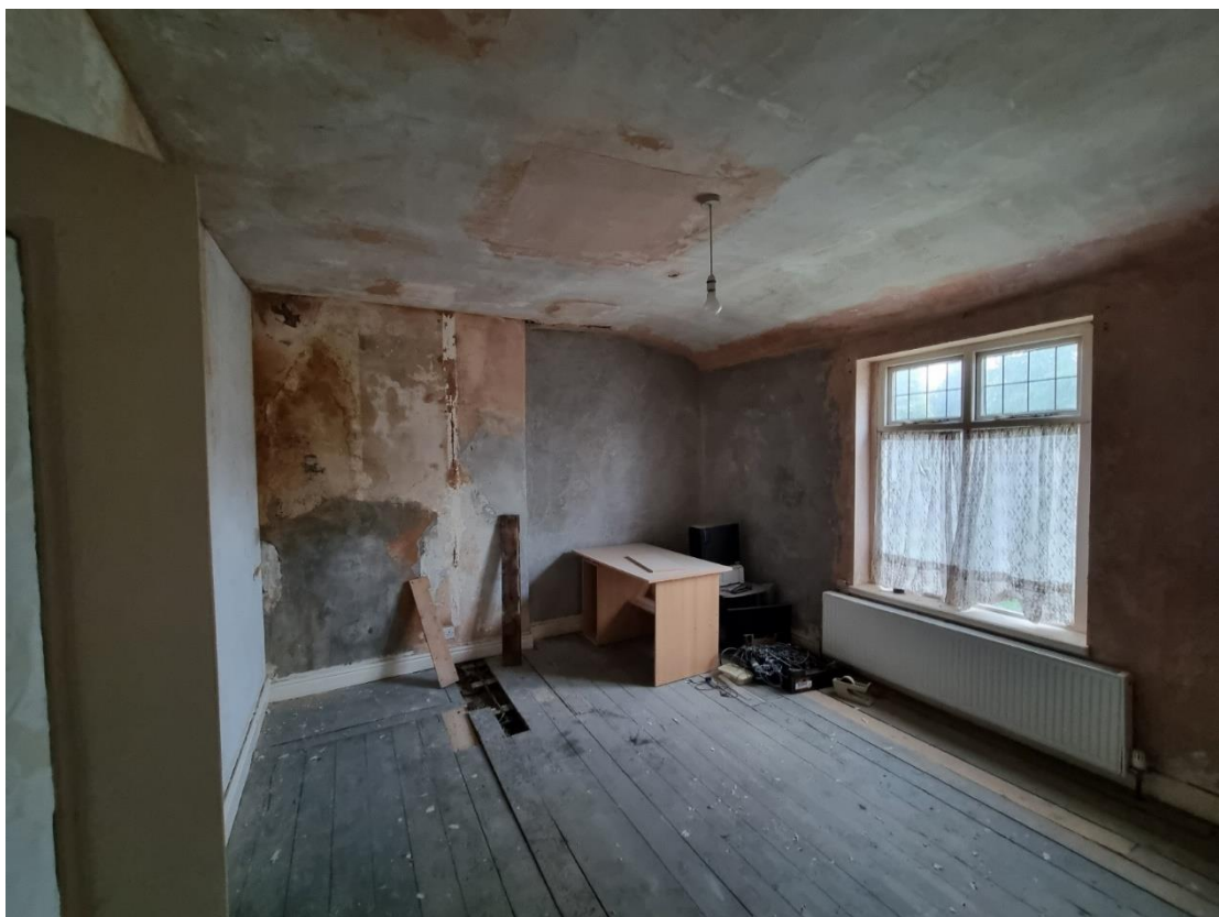
Fig.35: Red circle denotes an area of gypsum plaster to be removed following water ingress. The area is to be allowed to fully dry out before lime plastering.
