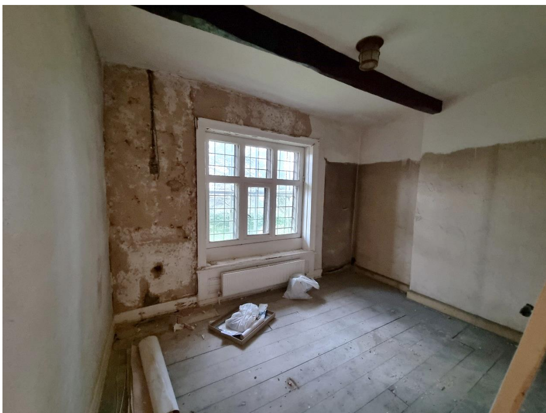
Fig.37: Failed modern plaster in bedroom 7 requiring replastering with lime.
