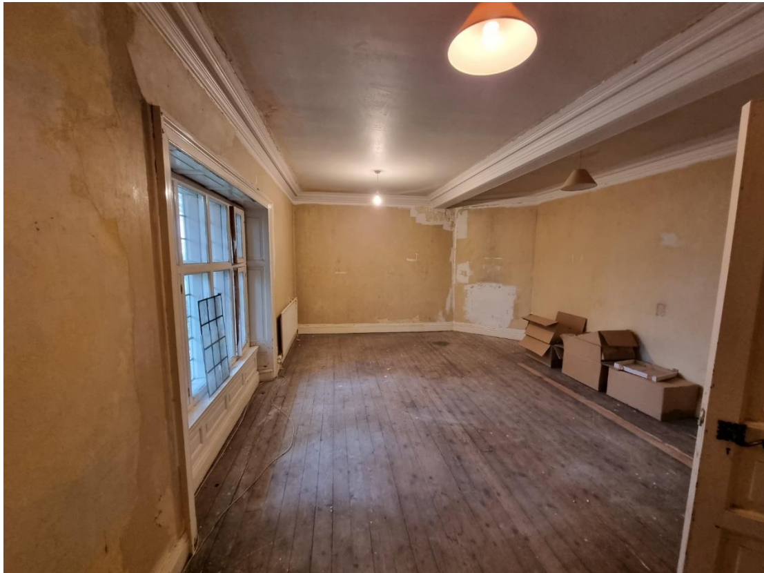
Fig.32: Bedroom 2, to be replastered with lime.
