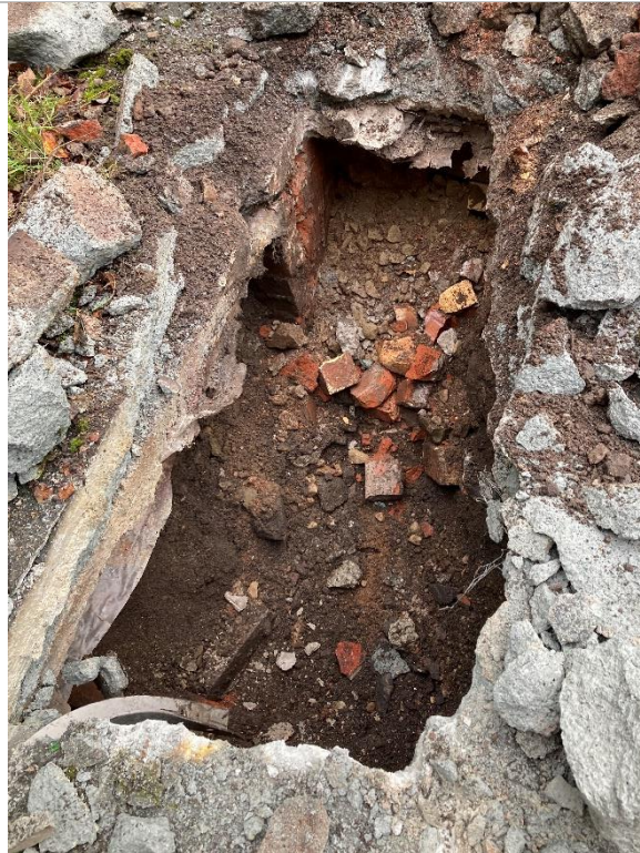
PLATE 5 TP107 EXCAVATION WITH OBSTRUCTIONS
