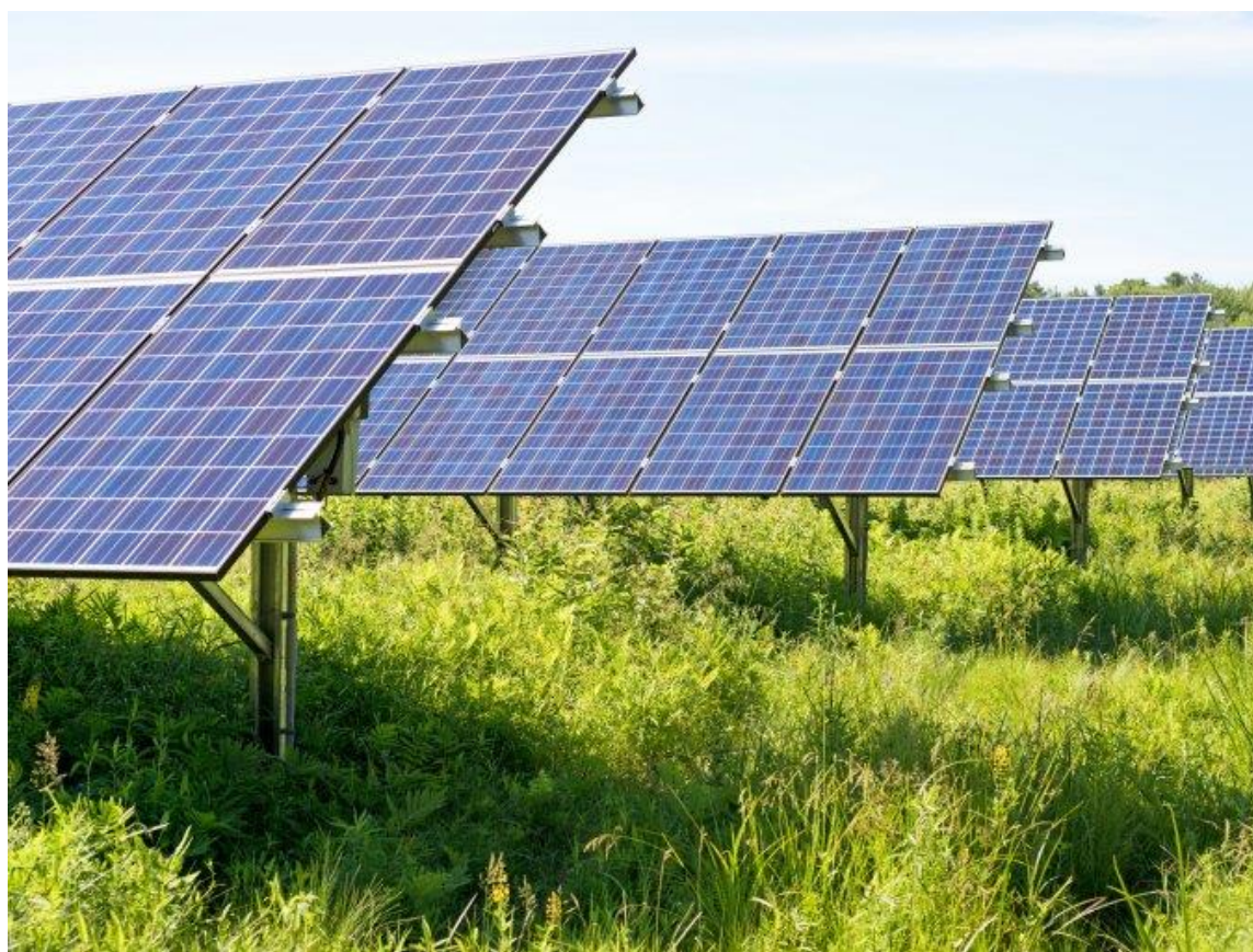
solar panel arrays screened from view by the building
