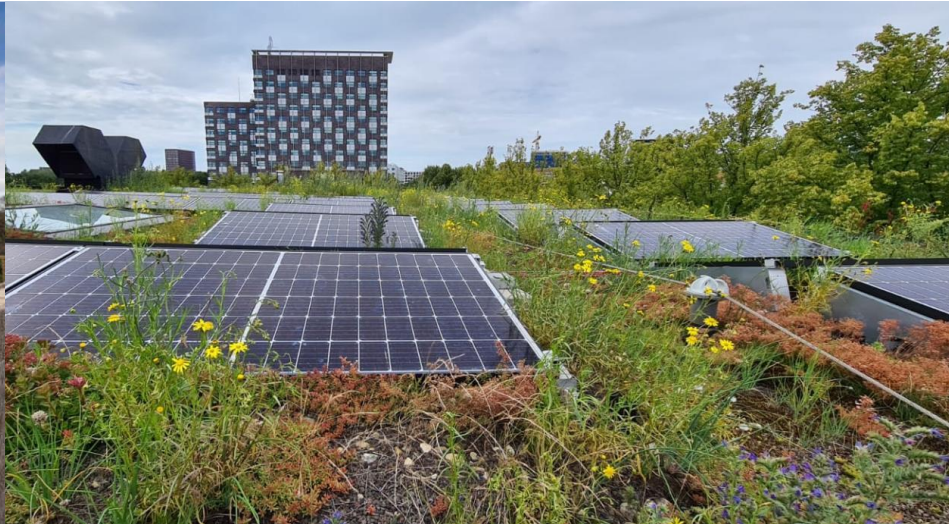
solar panel array above the garage-screened from view by parapet
