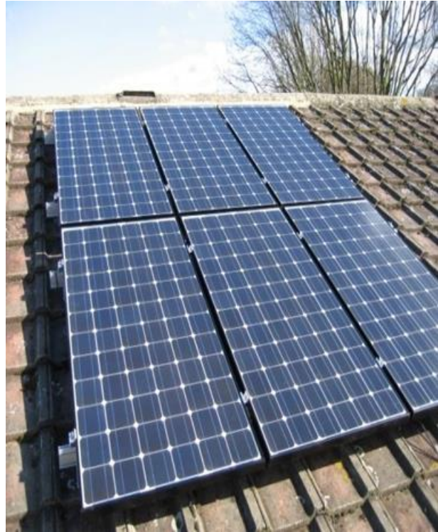
Figure 6 - Photovoltaic array on a pitched roof
