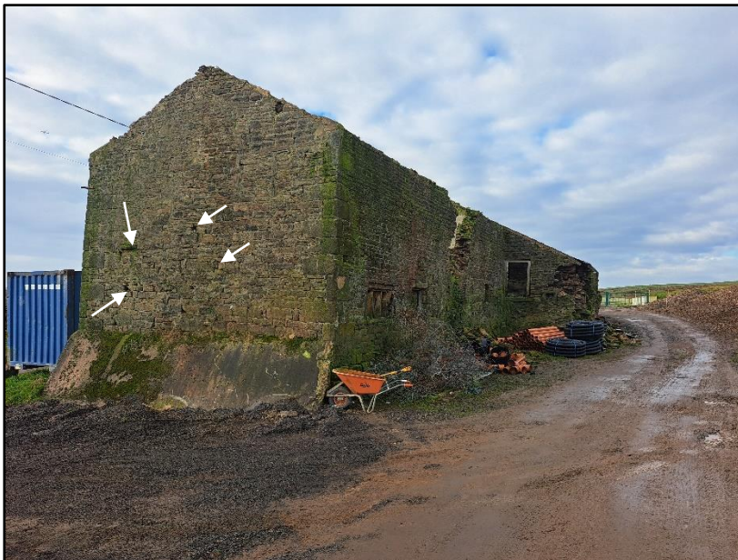
Photograph 4 showing crevices in the masonry (east elevation)
