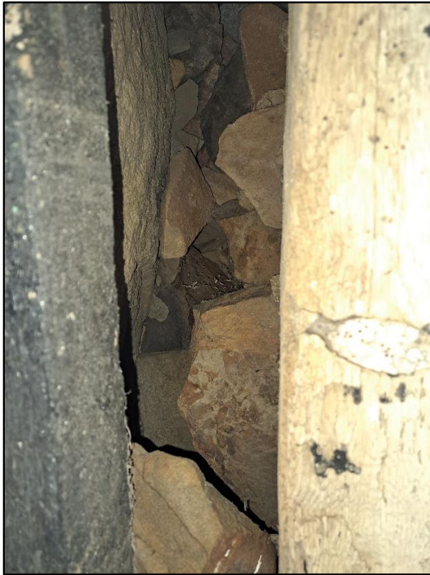
Photograph 5 showing a deep crevice in the masonry
