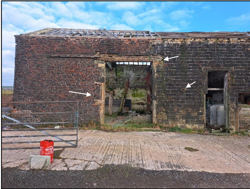
Photograph 3 showing crevices in the masonry (south elevation)
