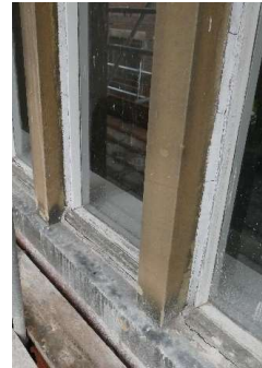
Meeting room windows uncovered to reveal areas of rot.
