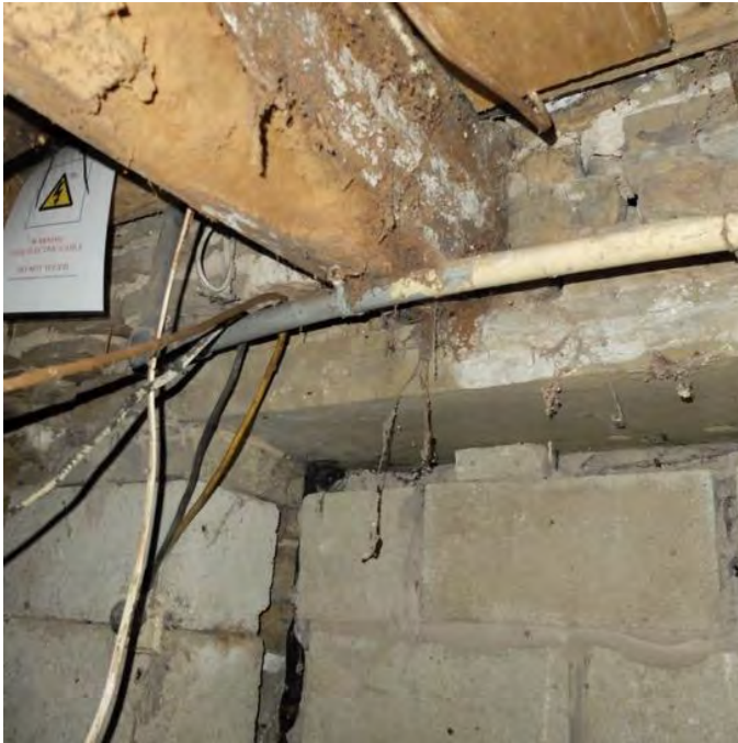
Photo. Decay to timber beam Room B1
