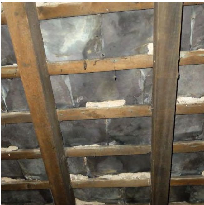
Photo. Slate fixings no underfelt. See original parging which has mostly fallen away.
