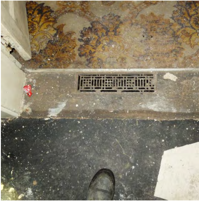
Photo. Vent to floor
