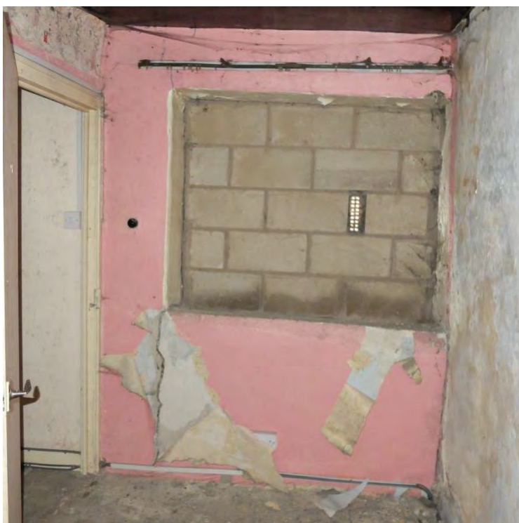
Photo. Cracking to below window west wall of outrigger Room F.07
