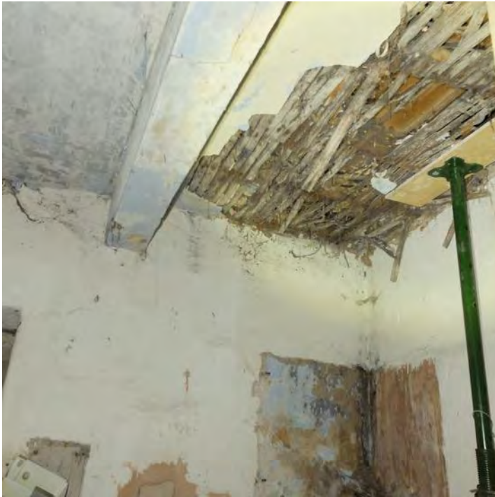
Photo. Example of damage to lath and plaster ceilings and downstand timber beam
