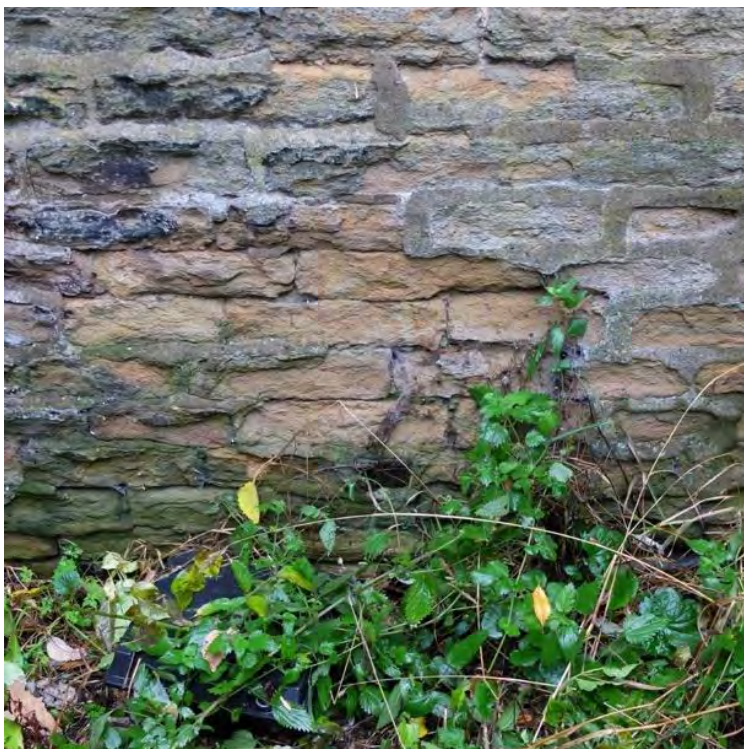
Photo. Corroded and frost damaged stone beyond repair.
