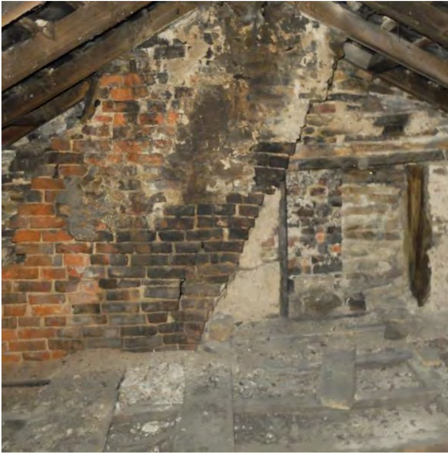
Photo. Crack at base of chimney the angle of build is too steep and urgent support is required, Roof space R1
