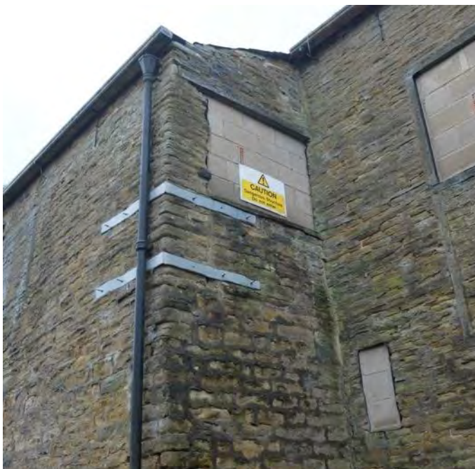
Photo. Outward bowing of wall caused by position of window opening.
