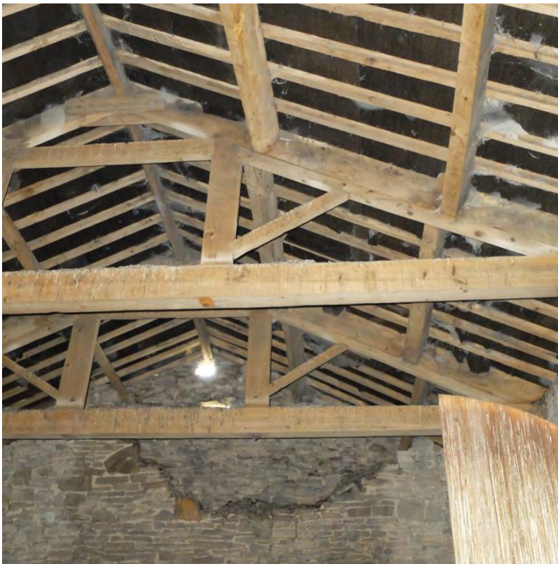
Photo. Collapse of inner leaf to gable.
