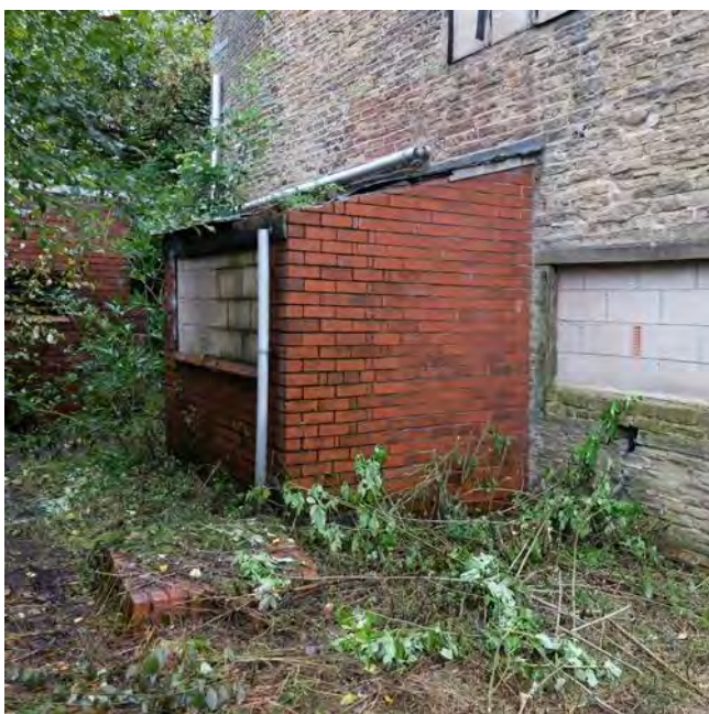
Photo. Brick porch, poor quality
