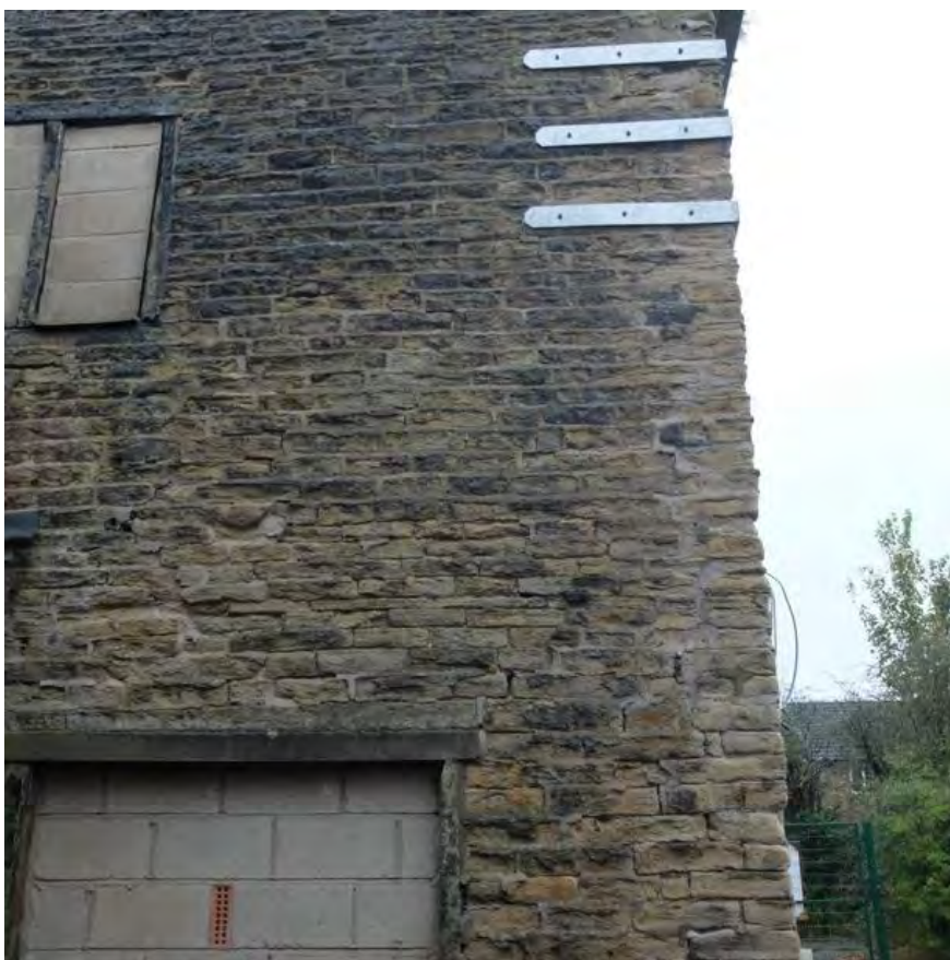
Photo. Frost damaged and eroded stone.
