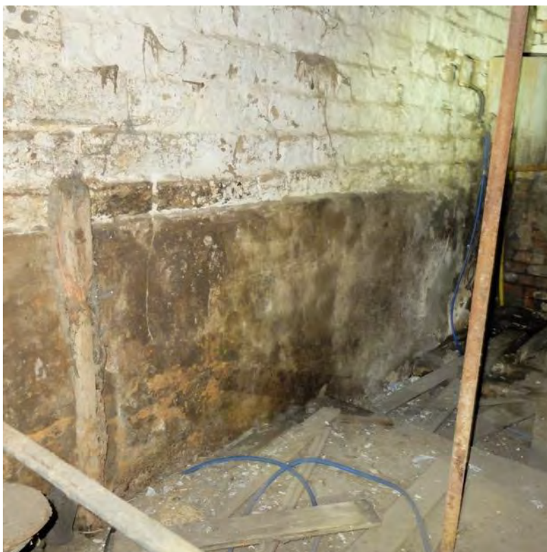
Photo. Tanking to external barn wall will be difficult to remove.
