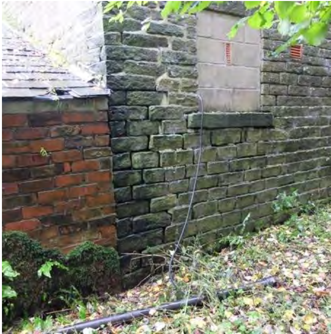
Photo. Loose brickwork at ground level
