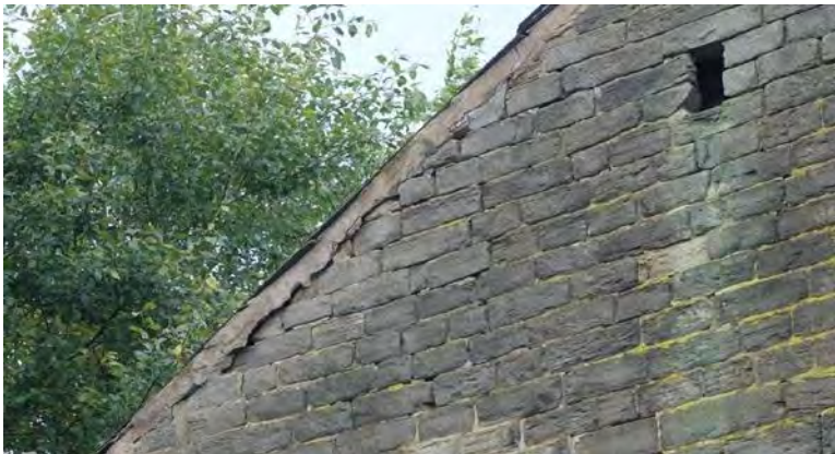
Photo. Loose cement verge pointing
