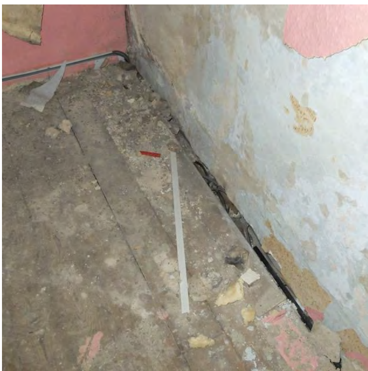
Photo. Gap between floor and wall indicates movement. Room F.07
