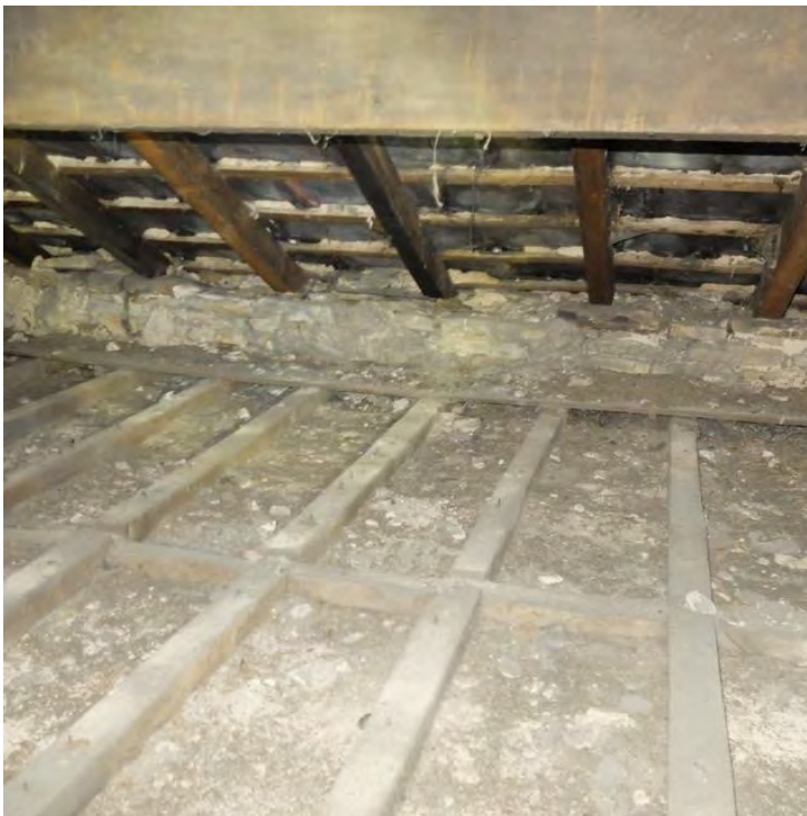
Photo. Rafters sit direct on wall head with no fixing down
