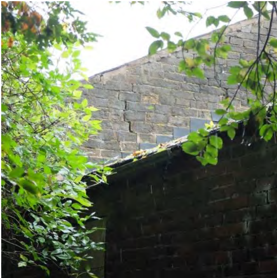
Photo. Movement extents up to roof level
