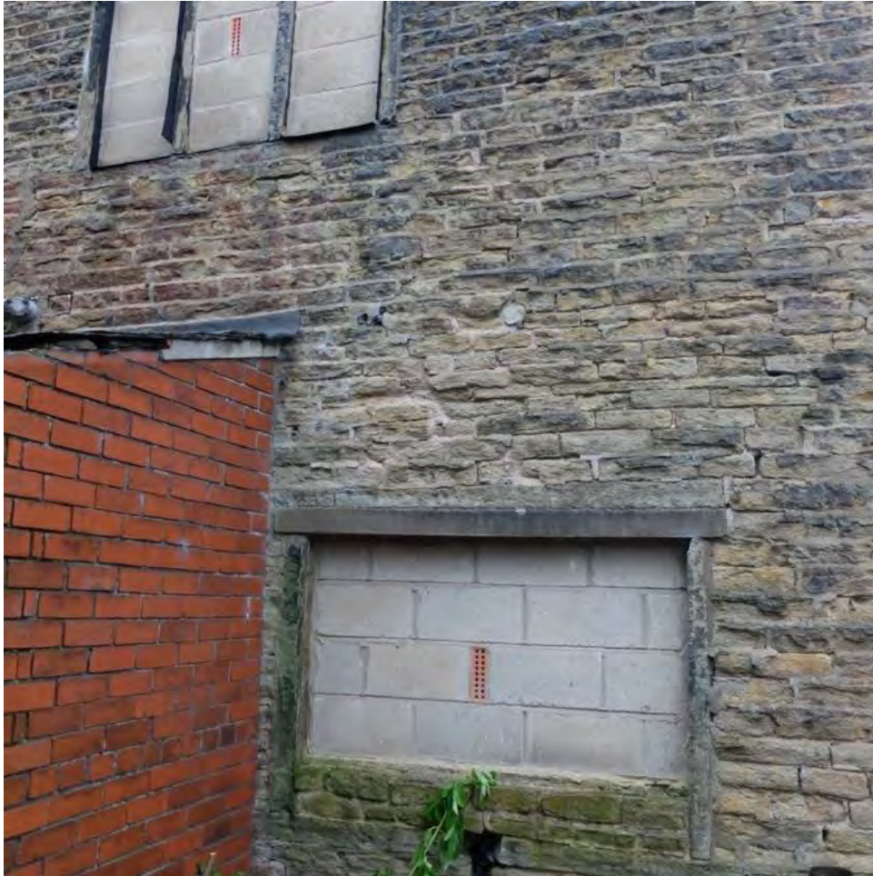
Photo. Cracking between ground and first floor windows.
