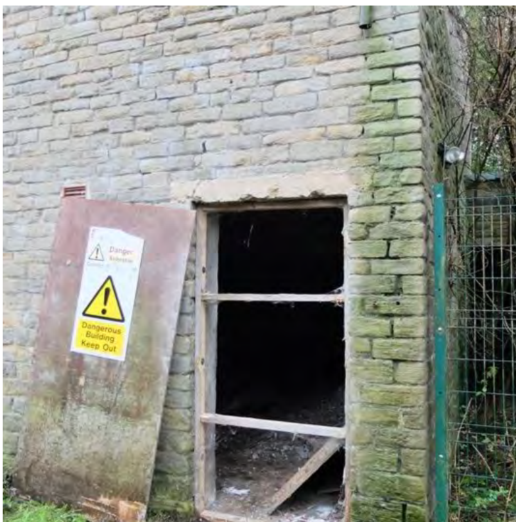
Photo. Damaged stone lintel above door
