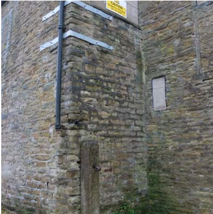
Photo. Eroded stone
