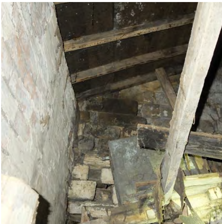
Photo. Movement above doorway which extends up to roof (photo above)
