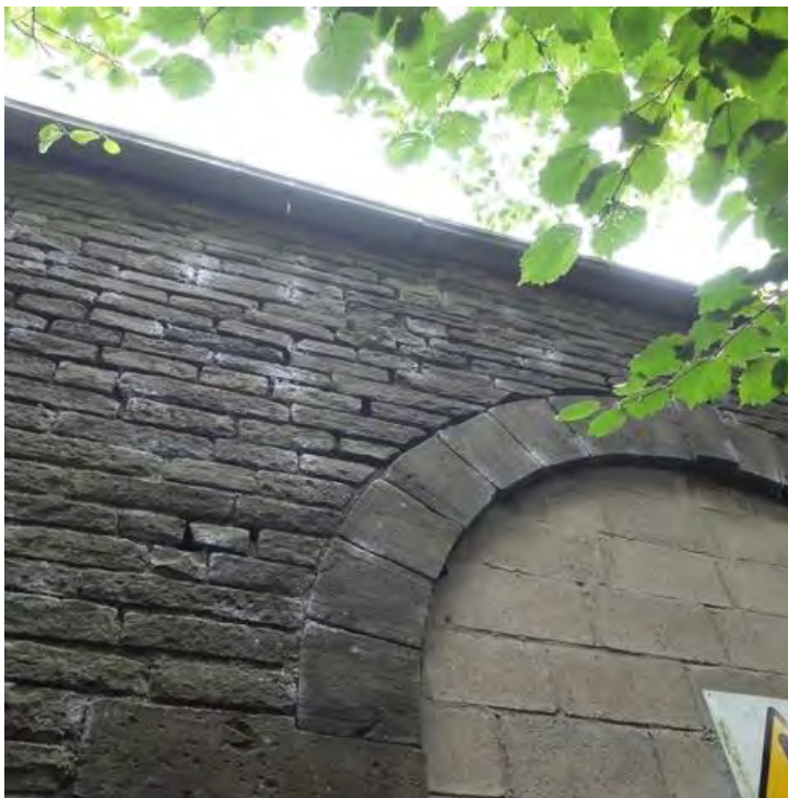
Photo. Mortar was away by leaks
