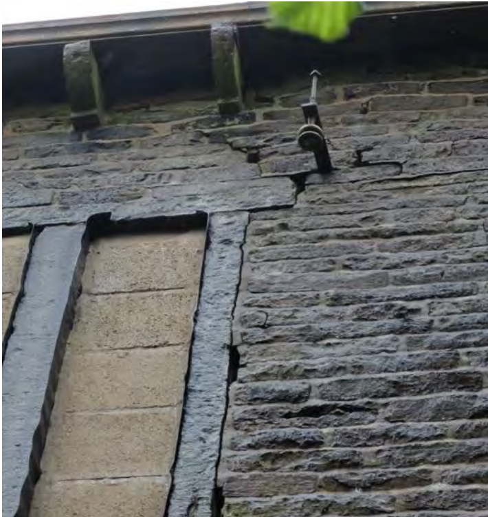
Photo. Crack from roof along vertical stone reveal to window.
