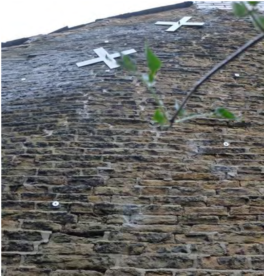
Photo. Bowed section of gable around flue to chimney.
