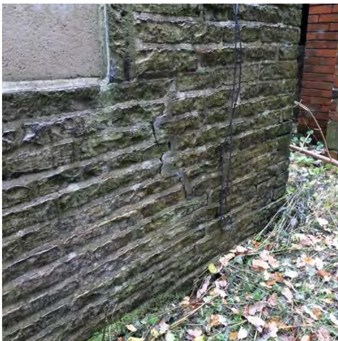
Photo. Diagonal cracking towards front right corner
