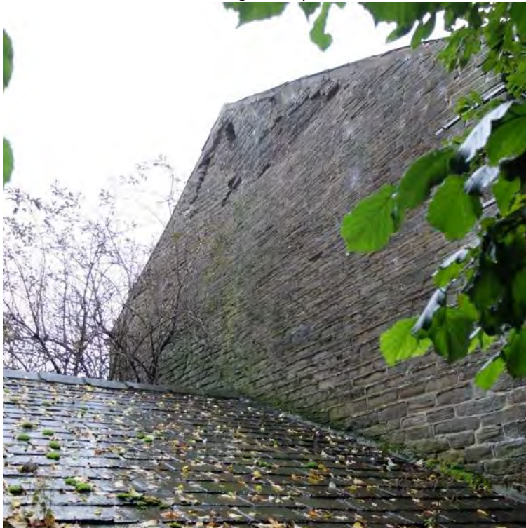
Photo. Inward bulge to high level gable
