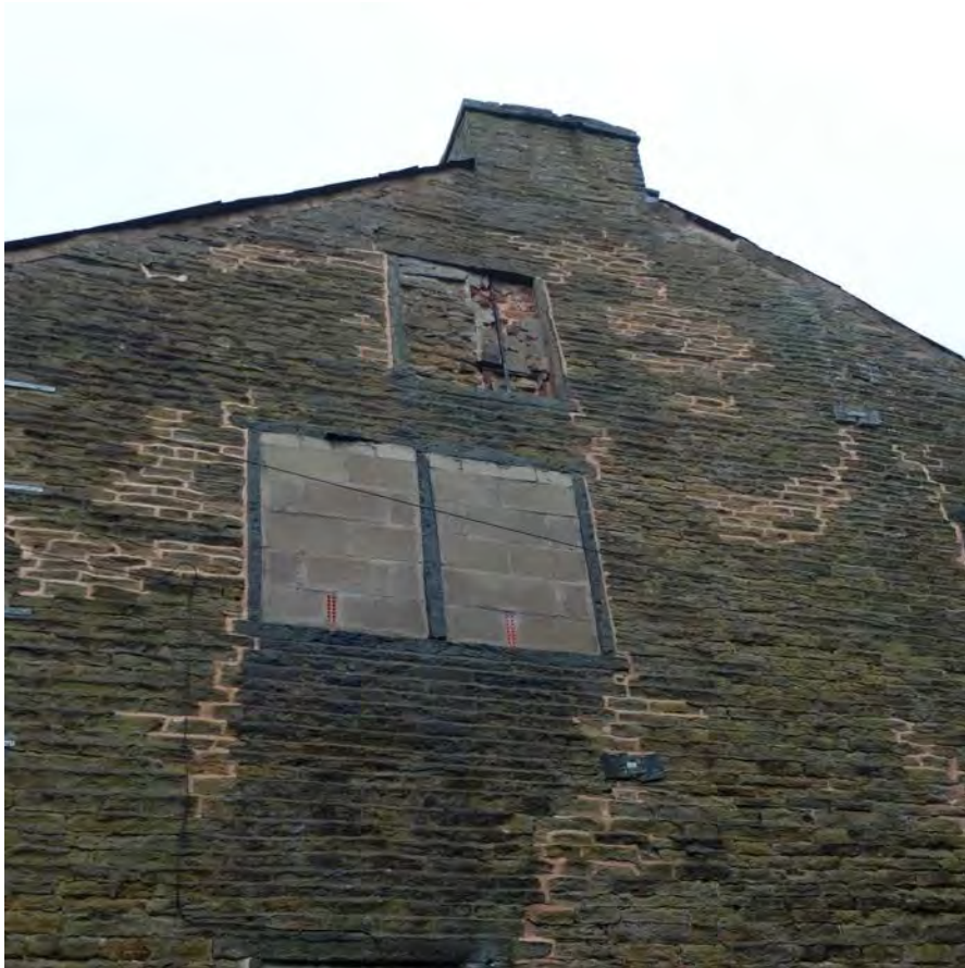
Photo. Previous repairs and bowing of masonry below chimney
