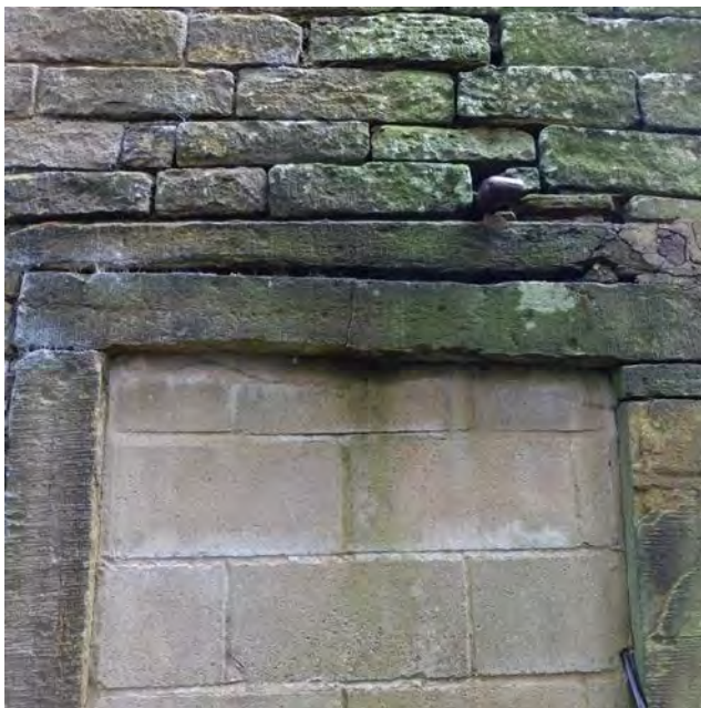
Photo. Crack to lintel and movement of masonry above
