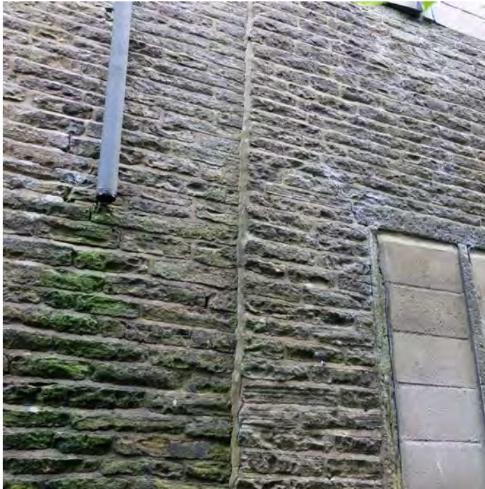
Photo. Outward bowing to extension wall at chamber level.
