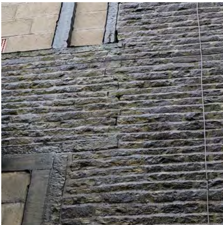
Photo. Crack extends from first floor to ground floor window.
