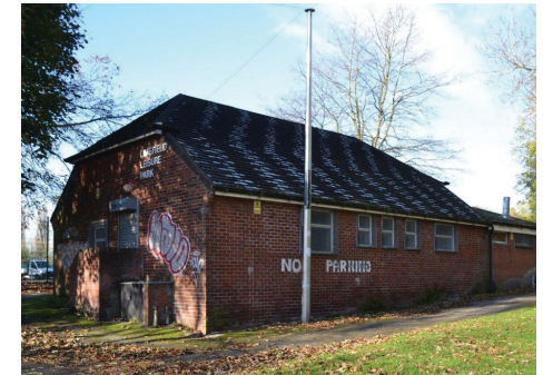
3. Limefield Leisure Park Utility Building - Showing signs of anti-social behaviour and a form (largely) through the hipped roof) at odds with the historic context.
