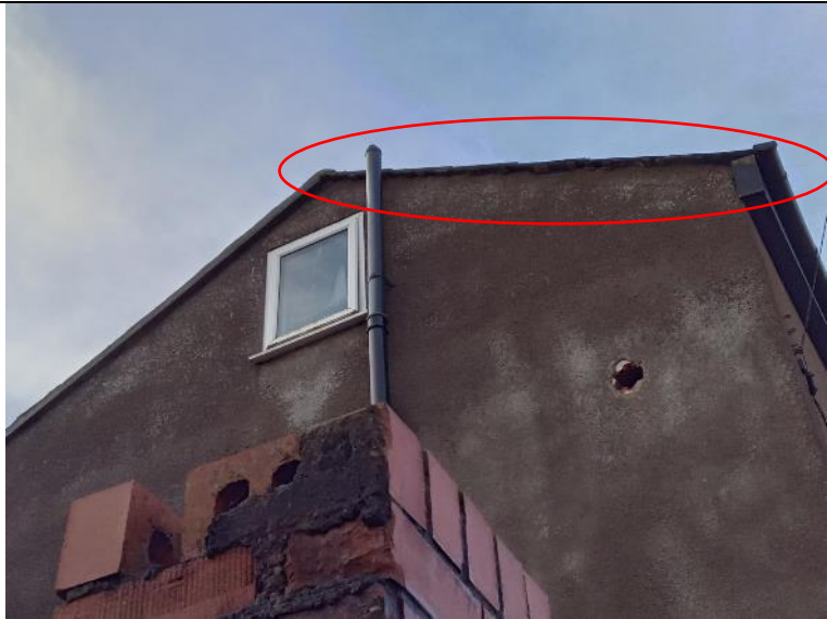
Figure 20. Eastern elevation – missing barge board.
