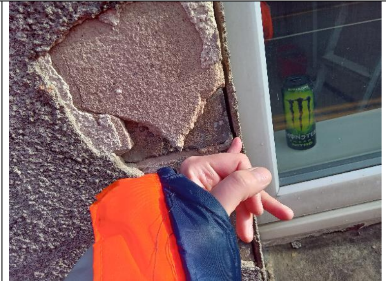
Figure 12. Western elevation – missing section of rendering.
