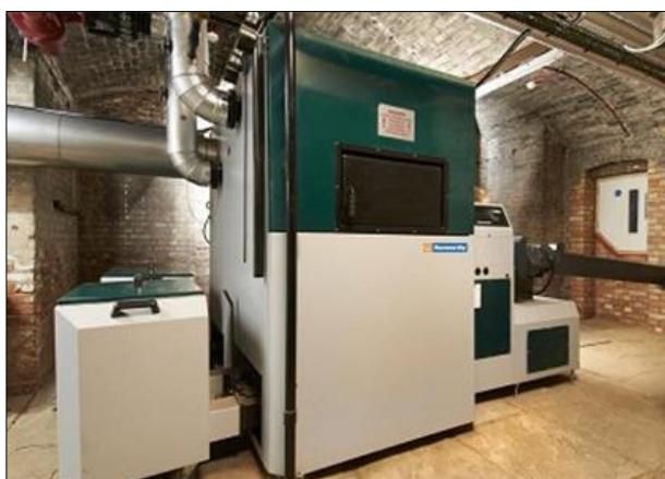
Figure 10. Commercial biomass boiler 4
