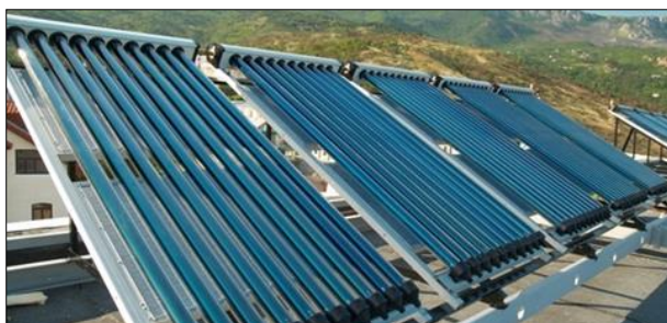
Figure 12. Evacuated tube solar collectors 6
