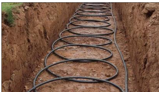
Figure 8. Horizontal ground loop collector 2
