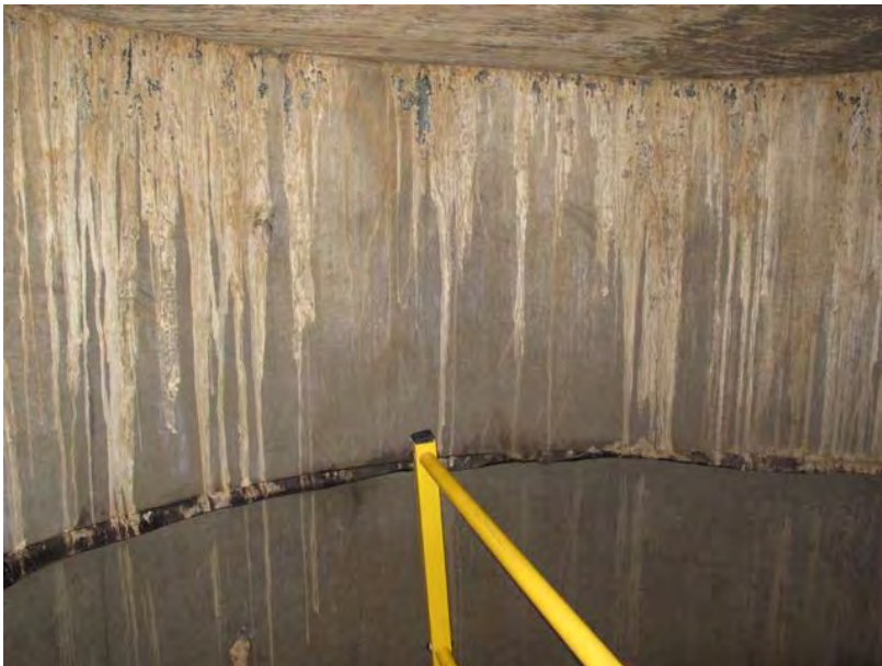
Views of Infiltration from Cover Slab at Level 1
