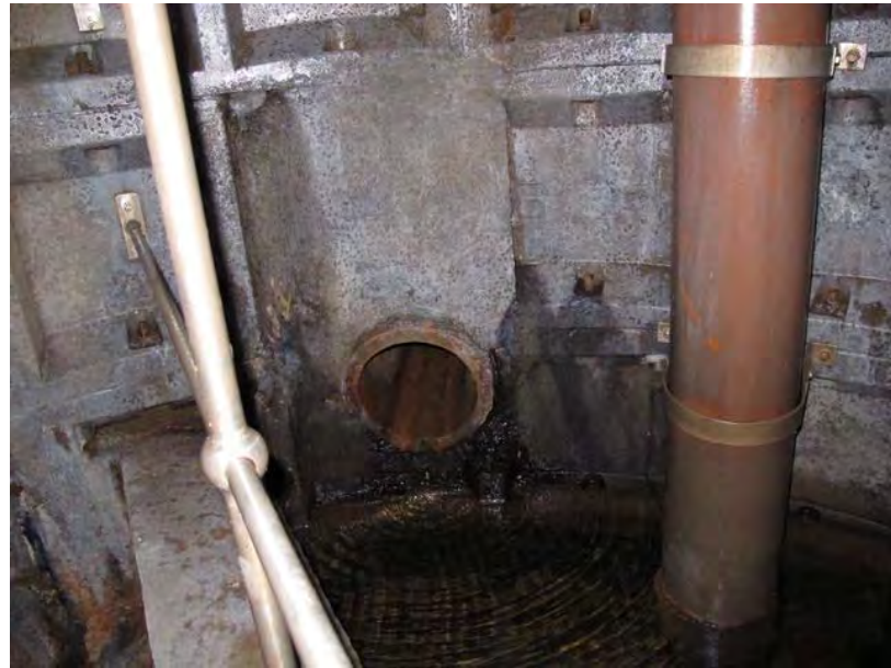
300mm Inlet Pipe into Sump and 225mm Drop Pipe.
