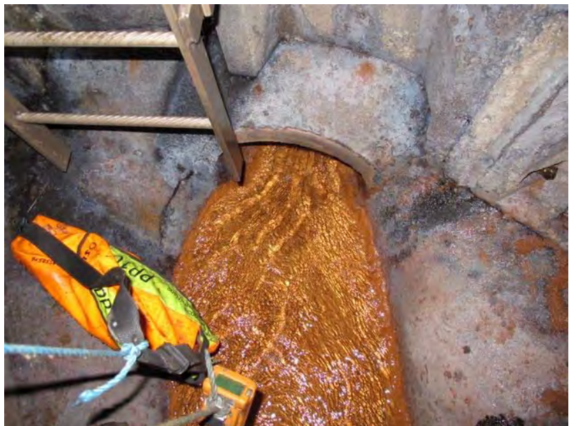
Foot of Ladder and Outlet Pipe at Level 3
