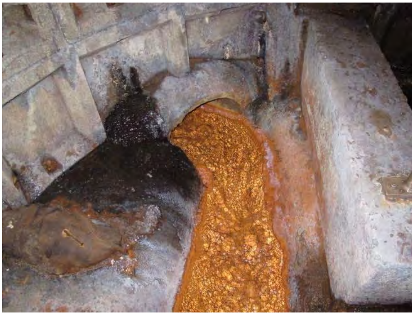
375mm Inlet Pipe and Channel
