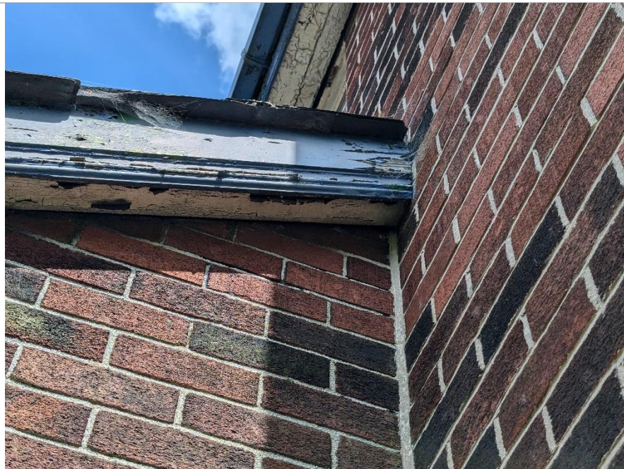
Photo 7. Gap under soffit on west elevation
