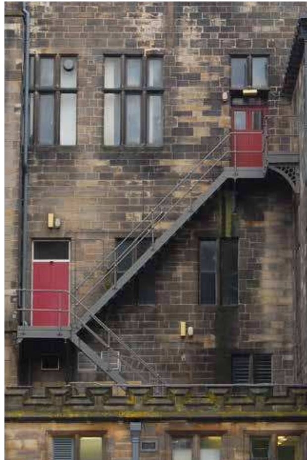
Later inserted fire escape to be removed and windows restored
