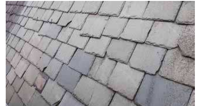
Existing slating to Great Hall Roof in poor condition
