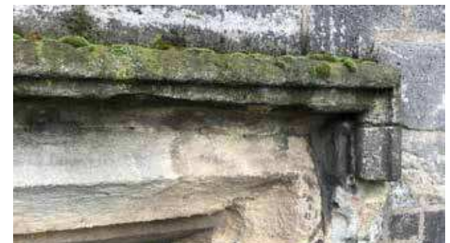
Example of eroding / failing masonry
