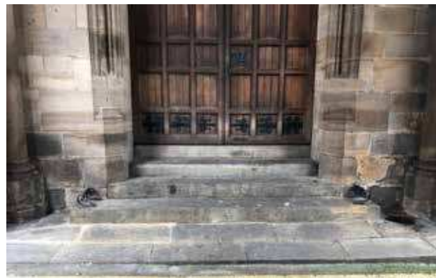
Stepped access to Mayor's Entrance to be overcome
