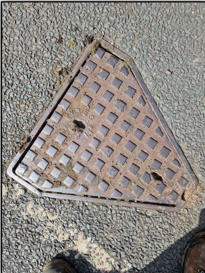
S2 Seized Manhole Cover
