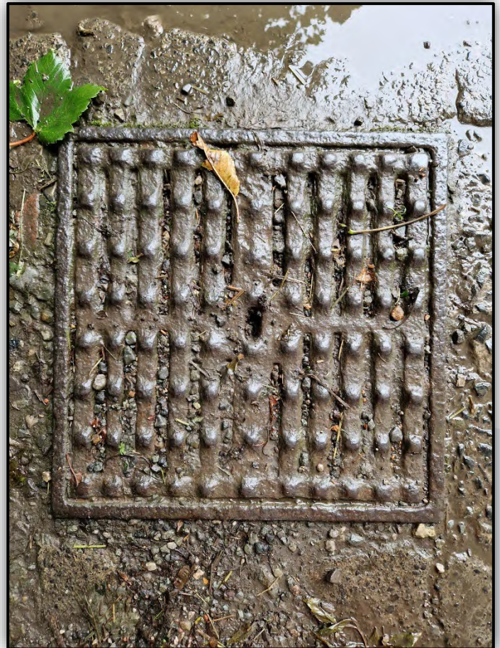
C5 Seized Grated Manhole Cover
